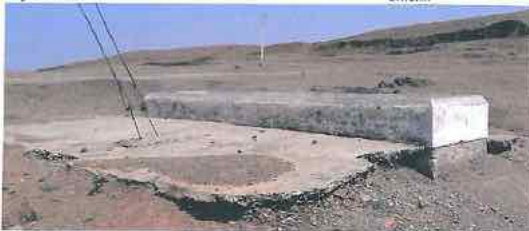
Achoda: Note the damaged platform.
