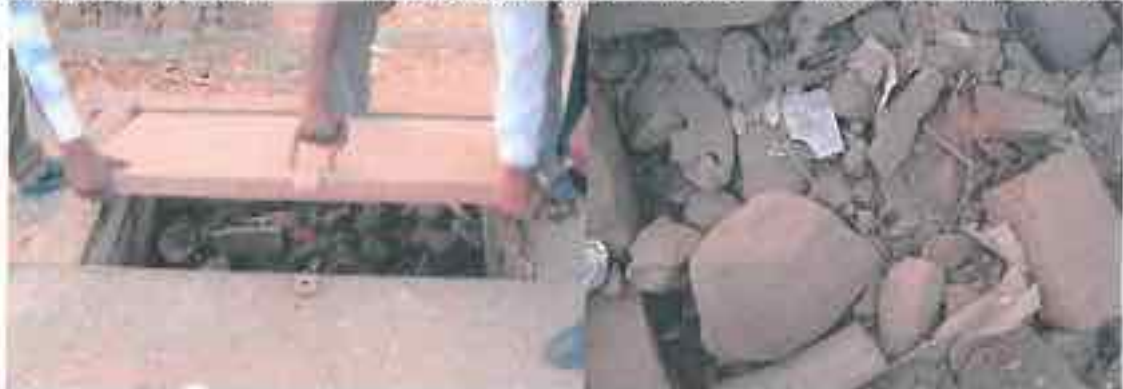
Bhilkheda: Inside of a Valve Chamber
