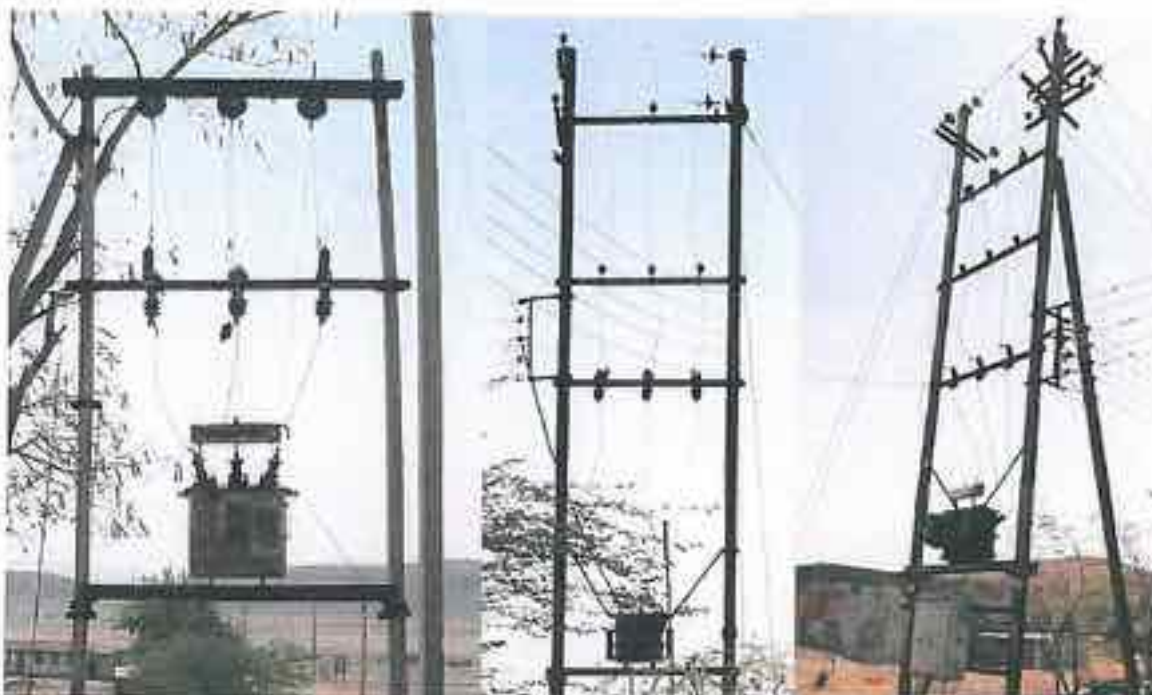
Missing Lightning Arrestors (Typical) at Dharamrai (Kukshi), Kadmal & Anjad Barda resp.
