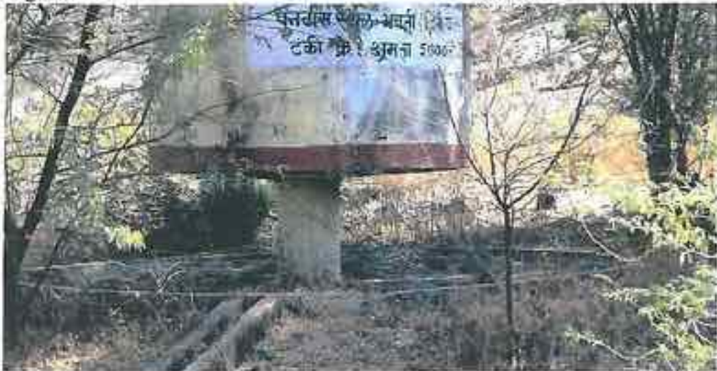
Bhawati-II: Mindless execution- the drain outlet channel lies at the base ring portion, while the opening of the ring portion does not drain into the drainage channel.
