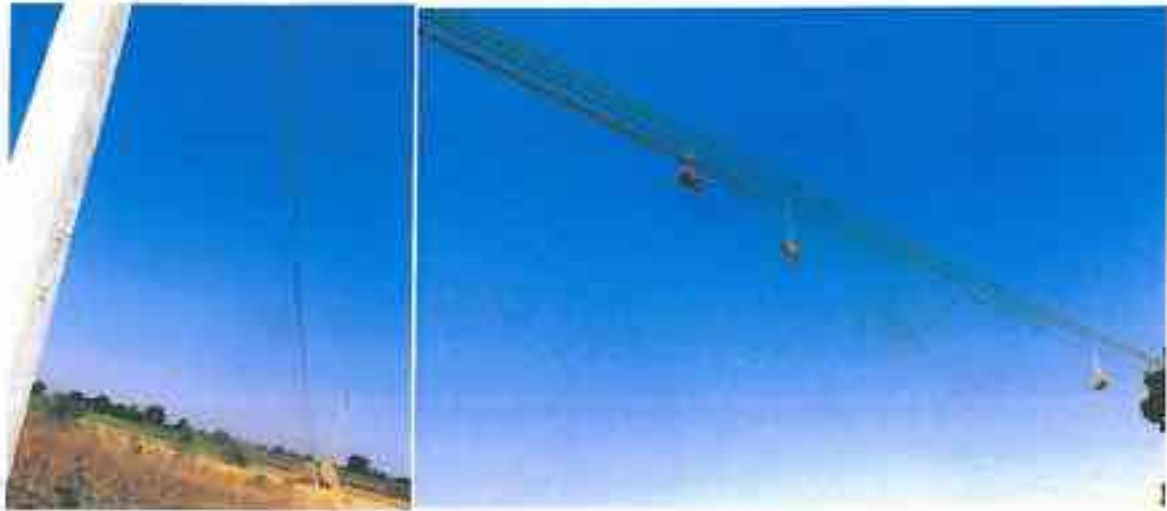
Plate 4.20. Chikalda: Loose Hanging Wires, absence of necessary gaps amongst the conductors compensated by hanging Bricks.
