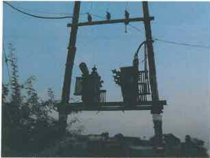
Nisarpur: One channel is missing above the Transformers, one of which is unconnected. AB Switch and Lighting Arrestors are missing. There is no LT Pole to separate out the 11 KV network from the LT Line. The cable is not seen supported by Metallic Bearer Wire.
