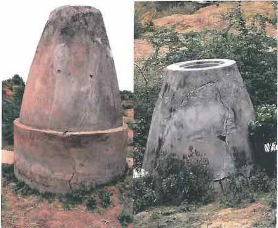
Plate 3.2.9. Dharampuri: Typical Huge sewerage manholes presumably in the low-lying area prone to flooding. Note the large Longitudinal Cracks, and extensive damage. Very poor execution and work supervision.
