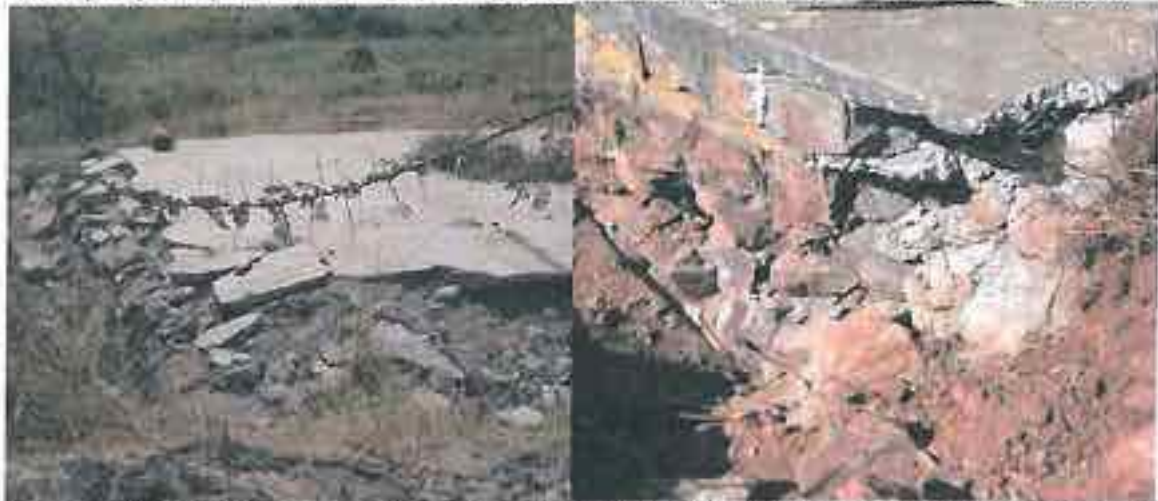
Poor quality and collapse of Tree Platform at Khalbujurg (left). Poor masonry joints and vertical cracks at a tree platform at Amlali.
