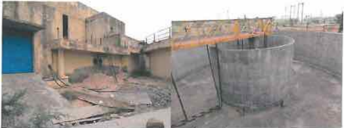
Ganpur (Manavar): Incomplete Water treatment plant works
