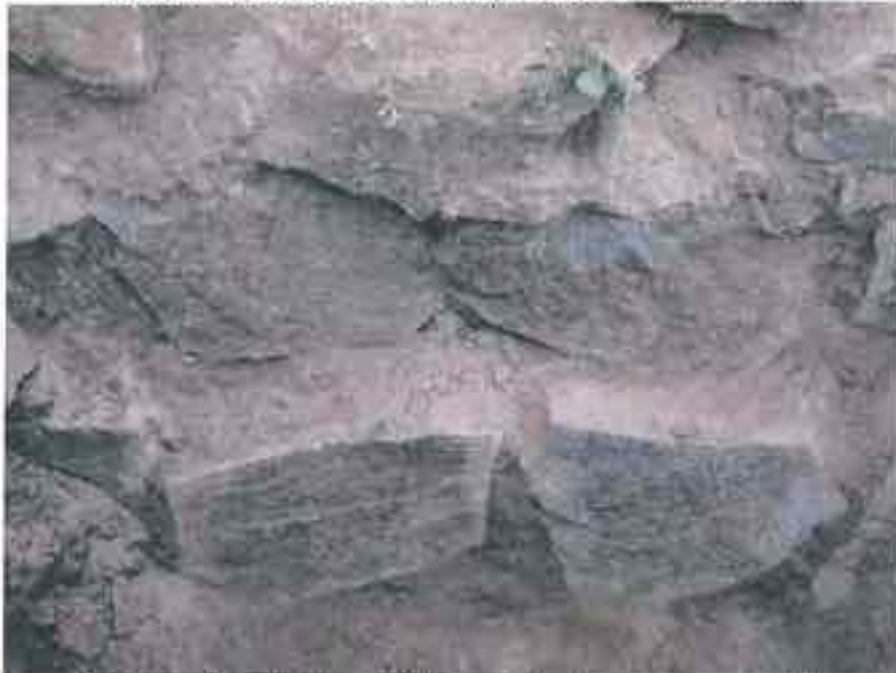
Nisarpur: Foundation at Primary School-poor wormanship
