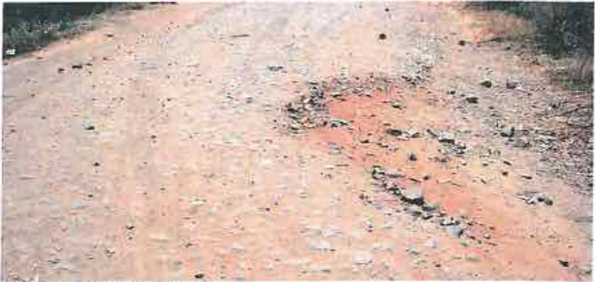
Raswa Deb: Typical Road damages
