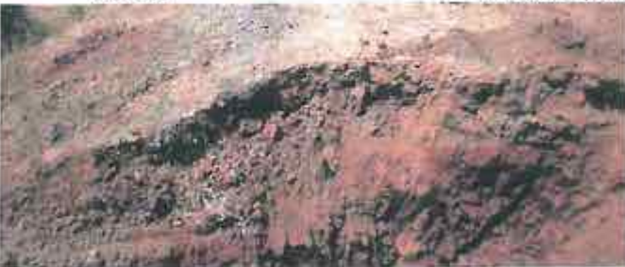
Jalkoti : A road cross section at a road collapse
