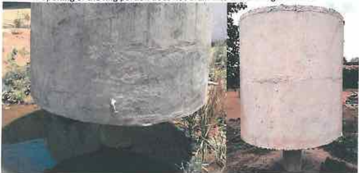
Vishwanath Kheda (Left) & Shakirpura (Right): Whitewash to hide massive cracks?
