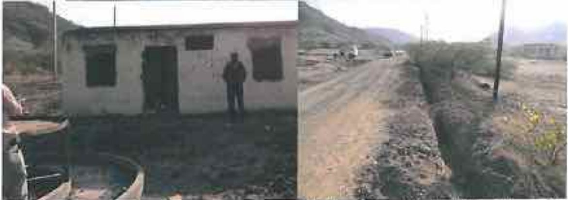
Plate 5.1 Abandoned Infrastructures at Sondul. The entire site, including the capital intensive Phase II Electrical Works, appears abandoned.
