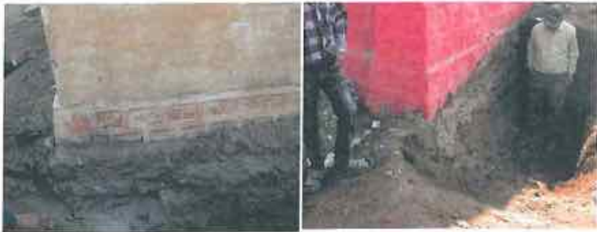
Bijasan: Aanganwadi located on sloping ground (left) had foundation depth 91-191 cm, whereas in similar sloping land, at the same site, the depth of foundation at Middle School (right) measured 76- 145 cm only.
