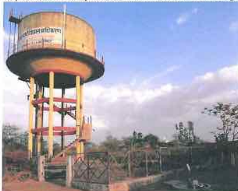
Chikalda: No provision of a Sump for 280 KL OHT. Also railing absent in part.
