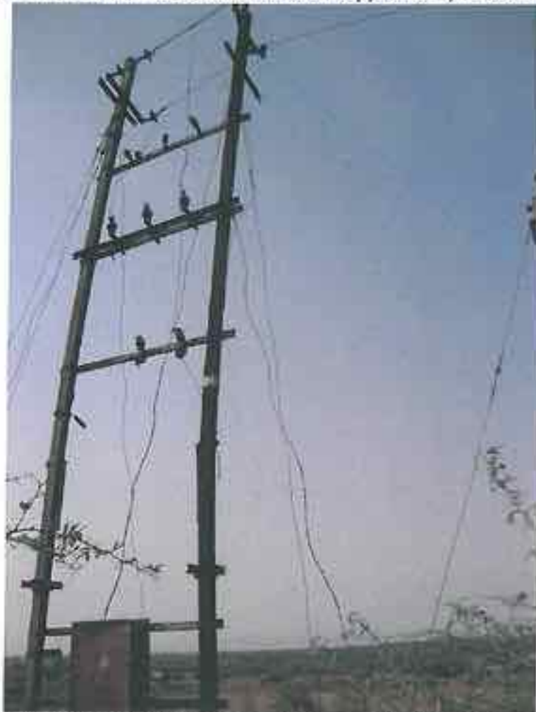
Poor mechanical strength of the Pole, Loose wires, Improper tightening of the overhead Conductors.
