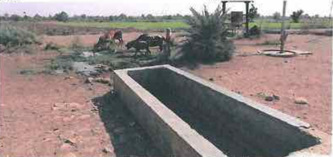
Chichli: Dry Halaos forces animals to depend upon pooled drainage from handpump spills. Plate 2.4.1. Dry Halaos - Infrastructure rendered defunct.
