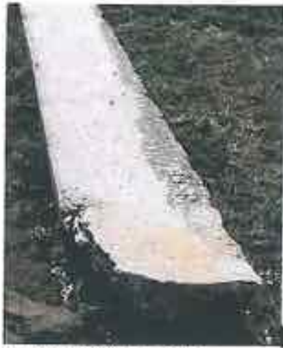
Nisarapur (A fallen Pole)
