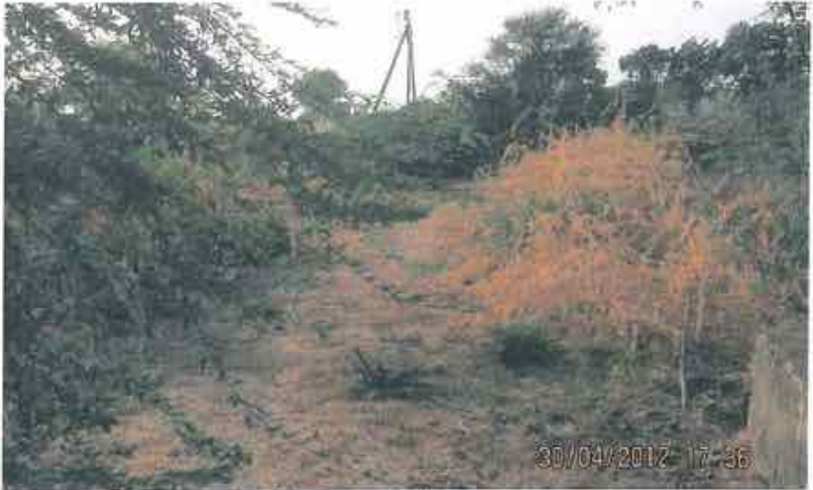
Saita: A road almost completely lost to vegetation
