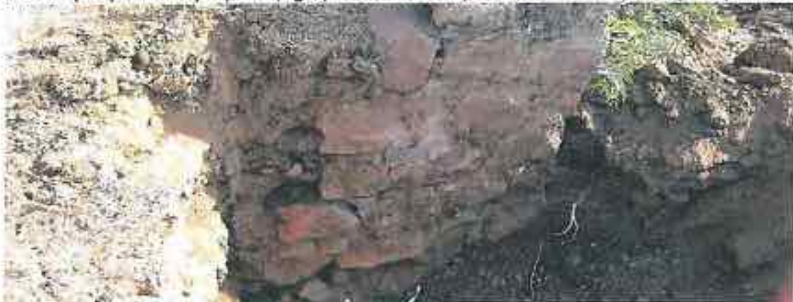
Bijasan: Foundation of RR Masonry culvert showing very poor joints
