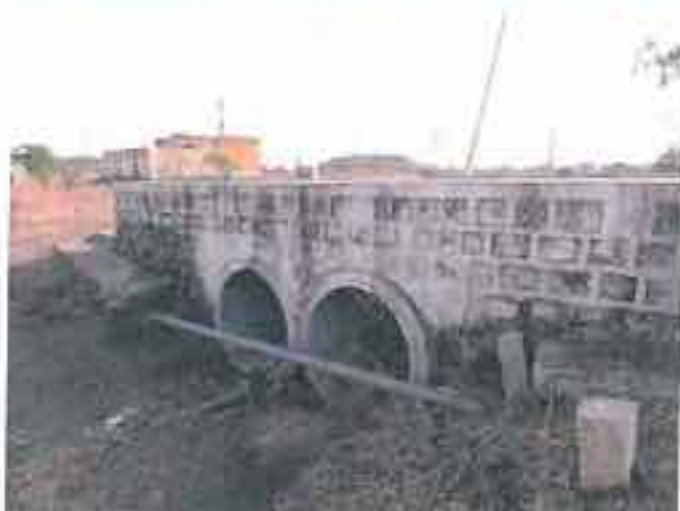
Gehalgaon : Careless Execution
