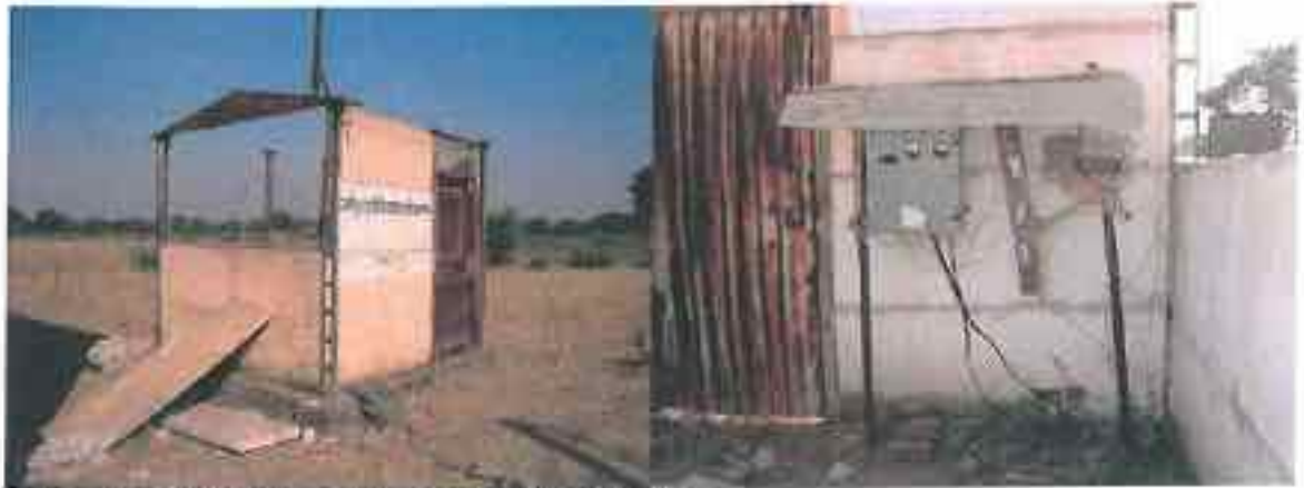
Kalyanpura: Outside and Inside the Pump House
