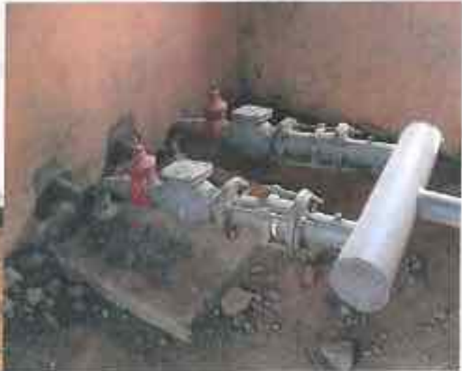
Awalda: Missing pumps imply OHT is defunct
