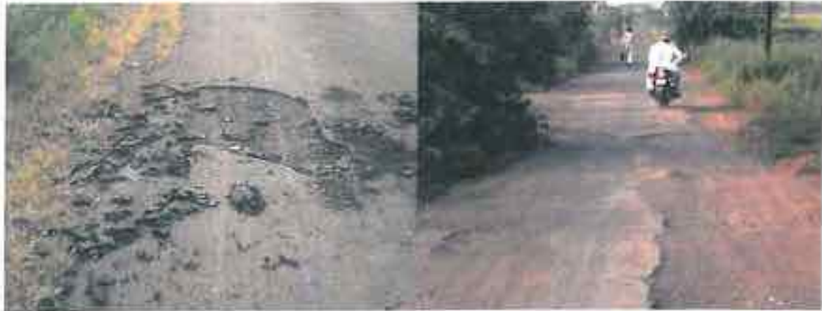
Nisrapur II/III: Poor roads, vegetation infested shoulders.
