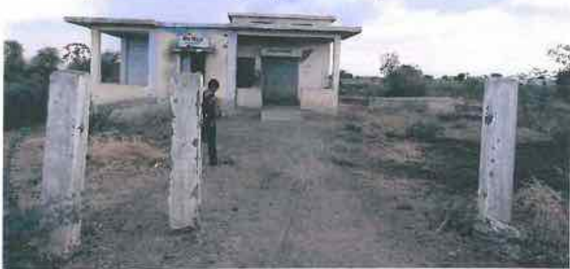
Moreghadi: Seed Godown- The access is higher, but the open area around the building has not been levelled, implying water will pool up during monsoons.
