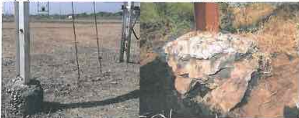
Borlai II (Phase II) : A recent 2009 Construction Note that the nearby pole has no muffing at all.
