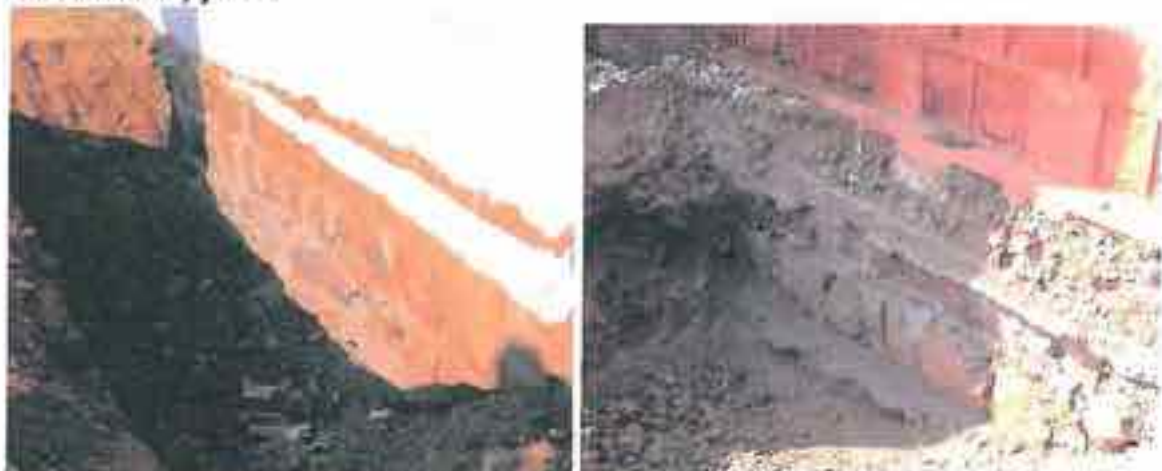
Poor masonry joints at Primary School Khedi (left) and Government High School, Dharamrai (right)
