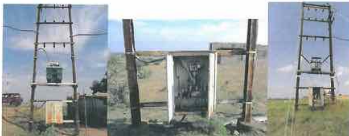
Plate 4.16. Three cases at Nisarpur : No lock and key arrangement, and No fencing around. Note the height of panel boxes in each case. Children would be tempted to open the boxes, and animals can be intrusive. Poor planning, execution, and workmanship.
