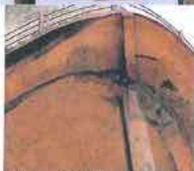
Sala: Signs of extensive leakage/seepage: Poor condition
