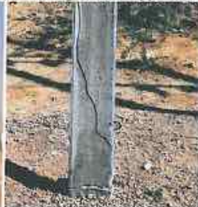
Borlai I: base crack & external earthing
