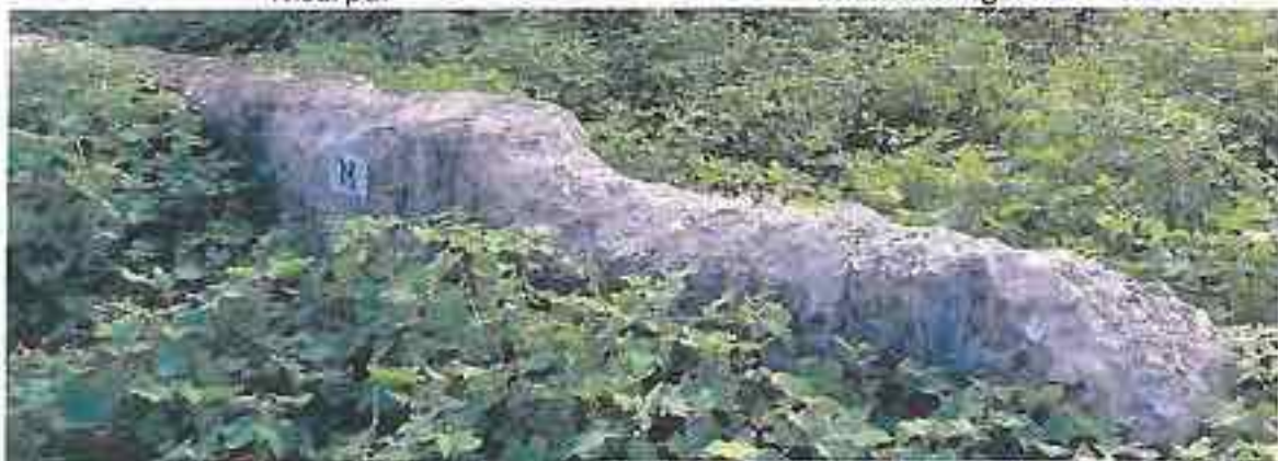
Umda: Poor concrete quality and construction
