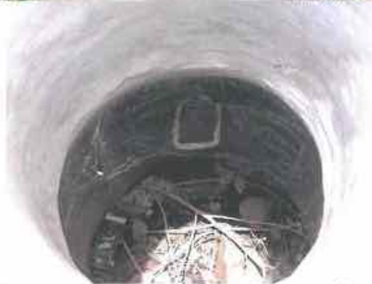
Plate 3.2.14. Dharampuri: Inside a Typical Deep Manhole – Sometimes just one or two footsteps provided even for deep manholes.
