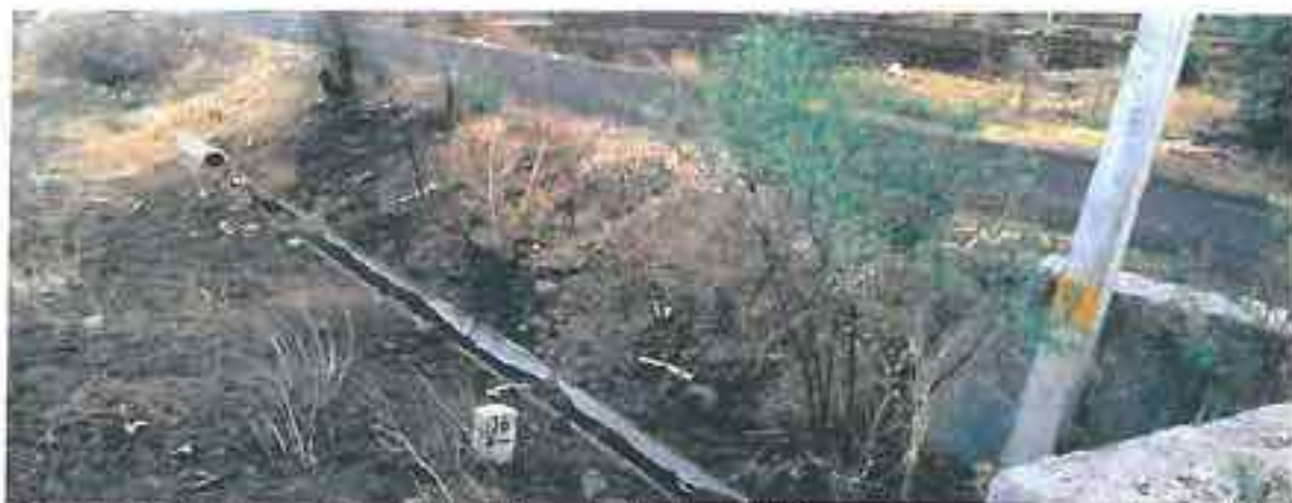
Moreghadi: Damaged shoulders. Also note the level difference between road top and the plot.
