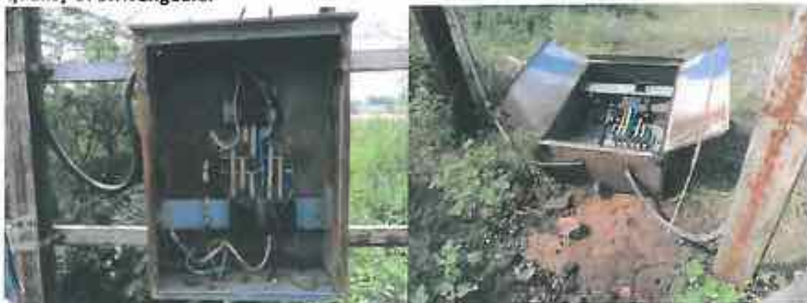
Plate 4.14. Two Panel boxes at the same site: Nisarpur, One without covers and Switch, and the other with covers, but lying on the ground, open, but with Switch. Thus differences in Panel quality were observed even at the same site.
