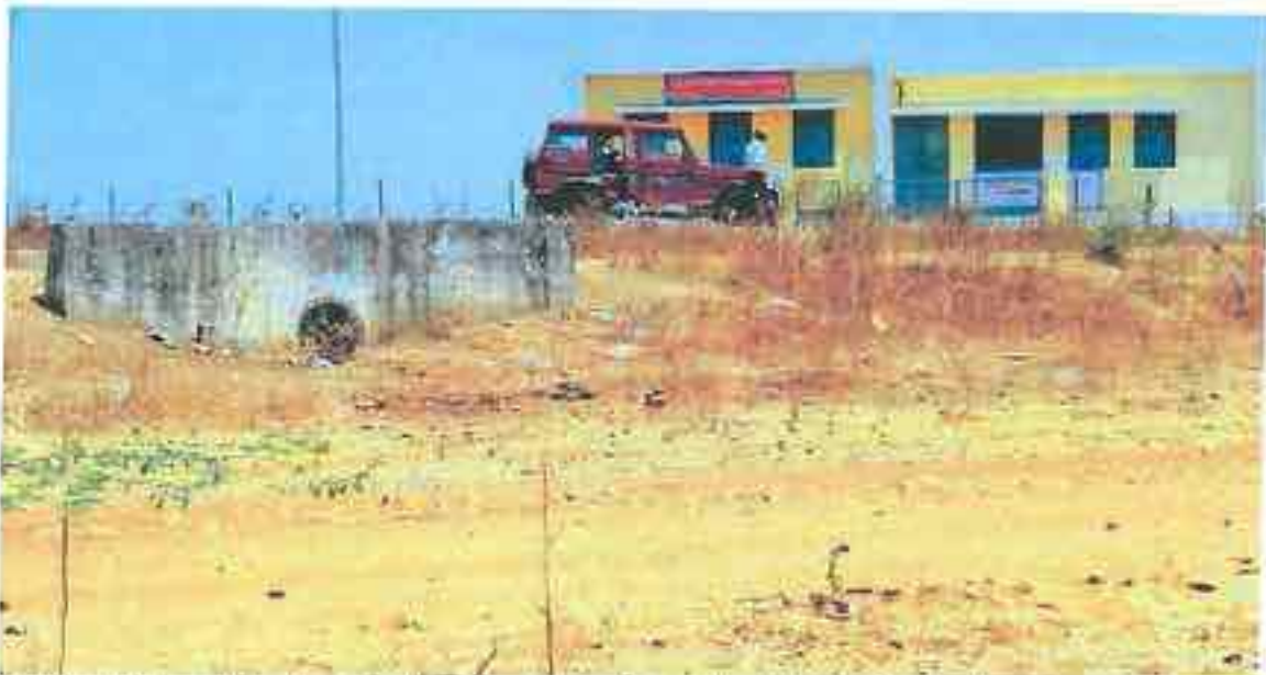
Gawla I: Culvert discharging directly on an oft used pathway: No drainage control
