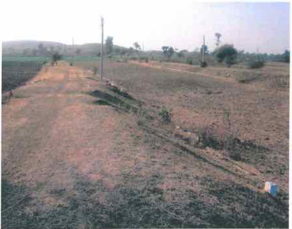
Chandankhed: Poor road condition, Poor condition of shoulders. Mark the position of the plot stone and electric pole. Note that there is no provisioning of street lights.
