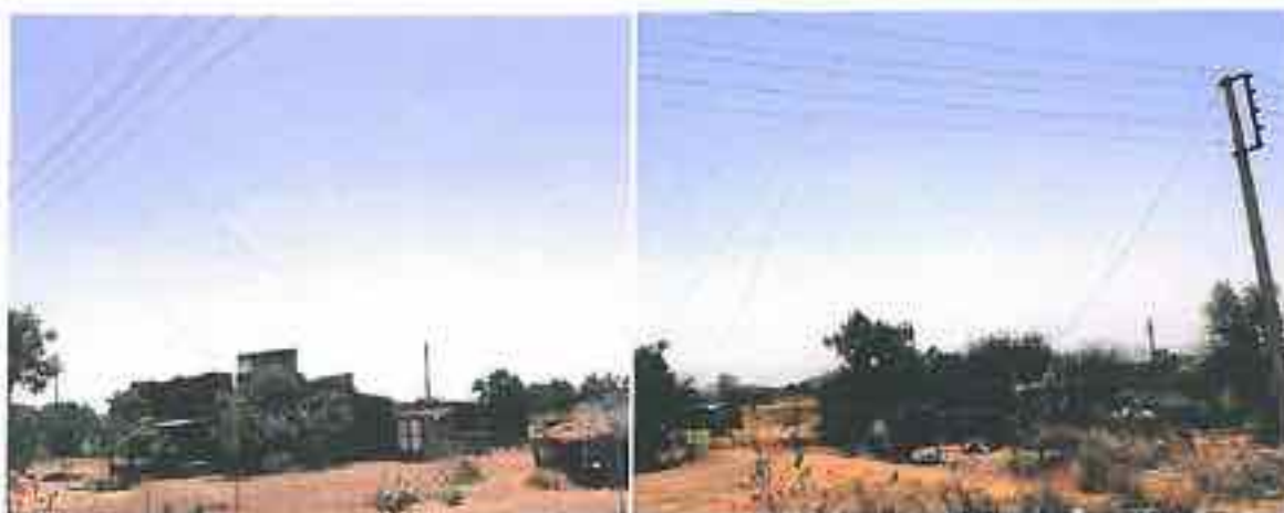
Plate 4.43. Illegal Connections thriving at Lakhangaon (Typical)
