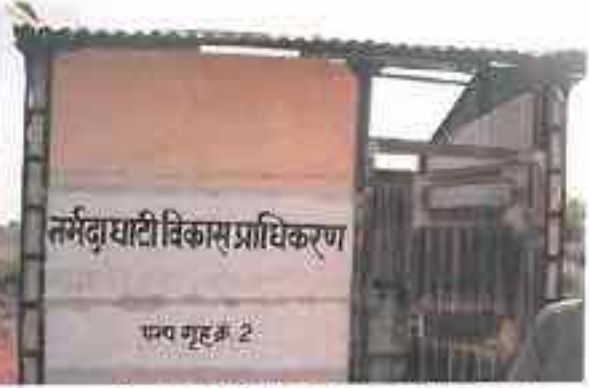
Borlai II: Part of the roof missing
