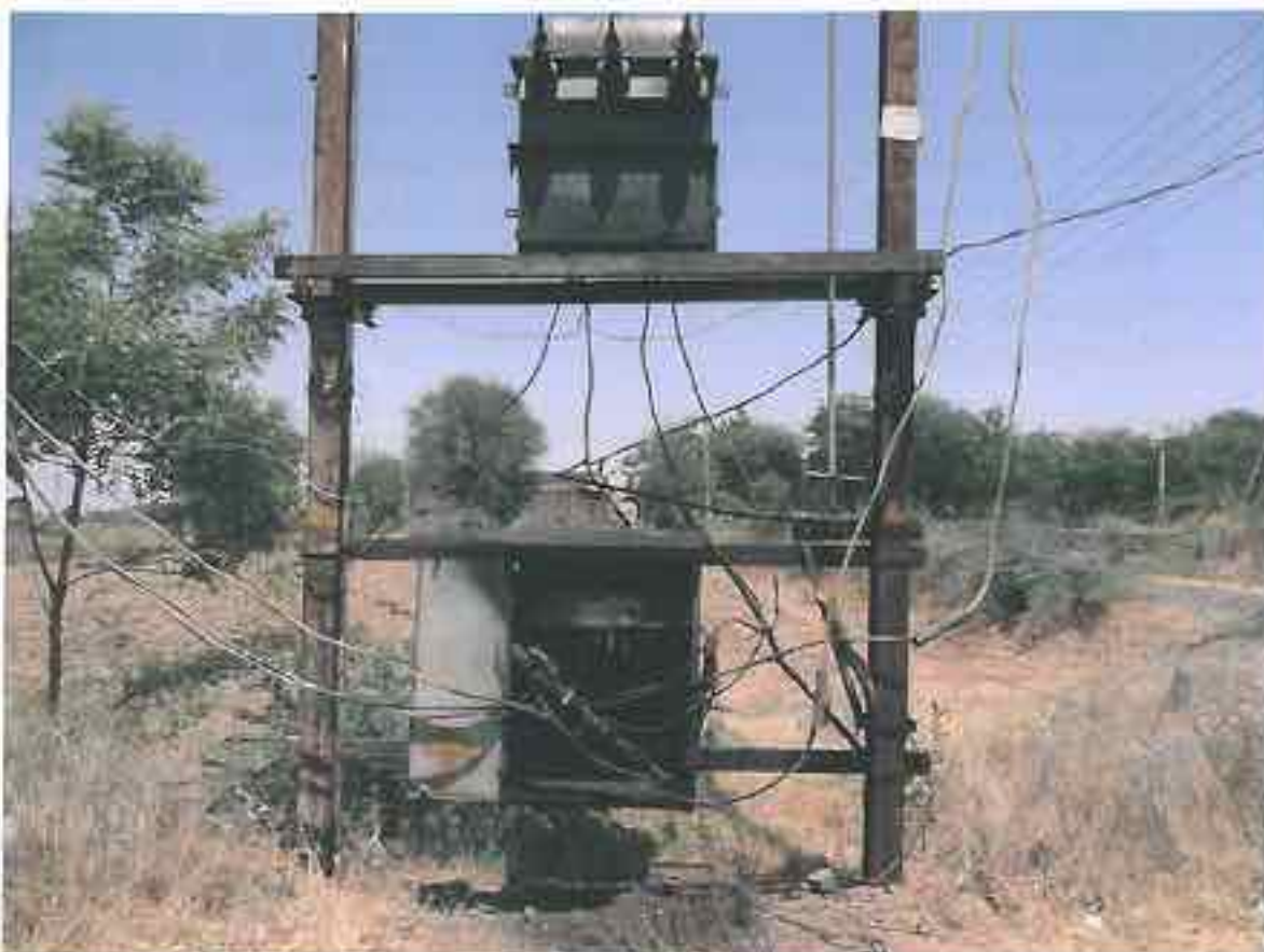
Sala: Highly dangerous and unsafe adhoc connections
