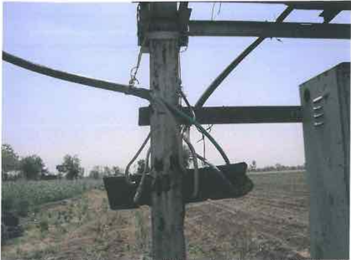
Semalda: Link Switch with Fuse and a Circuit Breaker Needed as per Rule 50 of the Indian Electricity Rules, 1956
