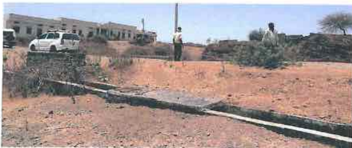
Chenpura: Drainage provided in parts only on one side of the road, and towards the lower side (building located on the higher elevation on other side of the road): This implies that the flowing water from higher slope is collected by the drainage system only after it crosses the road, and hence the road remains unprotected from the lateral flow of water flowing rapidly down the slope.
