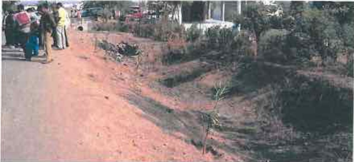
Kukra: Deep trenches upto 6 ft on both sides of the main approach road. Road safety jeopardised, more so as engineered side drains are non-existent (though culverts are present, but these are susceptible to silting and chocking up as engineered drainage is not present). What would happen in rains when ditches this deep stand filled up, and driver does not know where the road edge lies?
