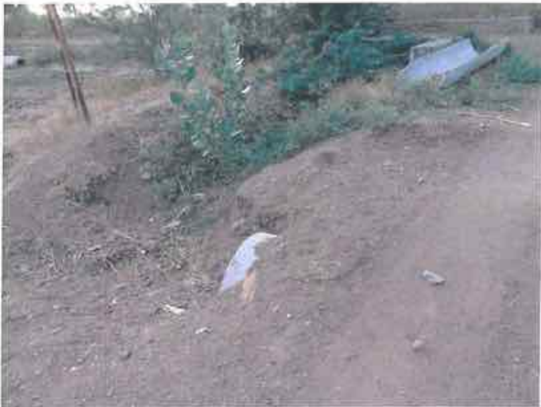
Ratwa –Adhoc pipe laid across the road for drainage with hardly any cover
