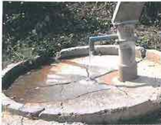
Khedi: Also the HP platform slope is defective
