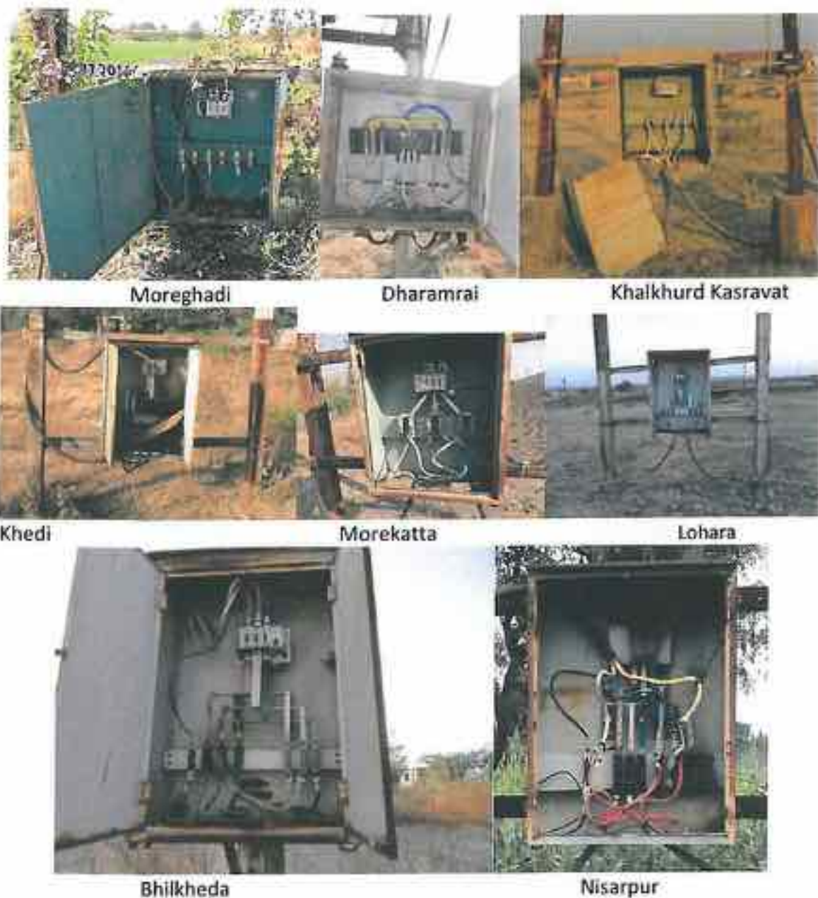
Plate 4.13: Safety Compromised: Missing Switches, Missing/unlocked covers, and Poor quality of switchgears.
