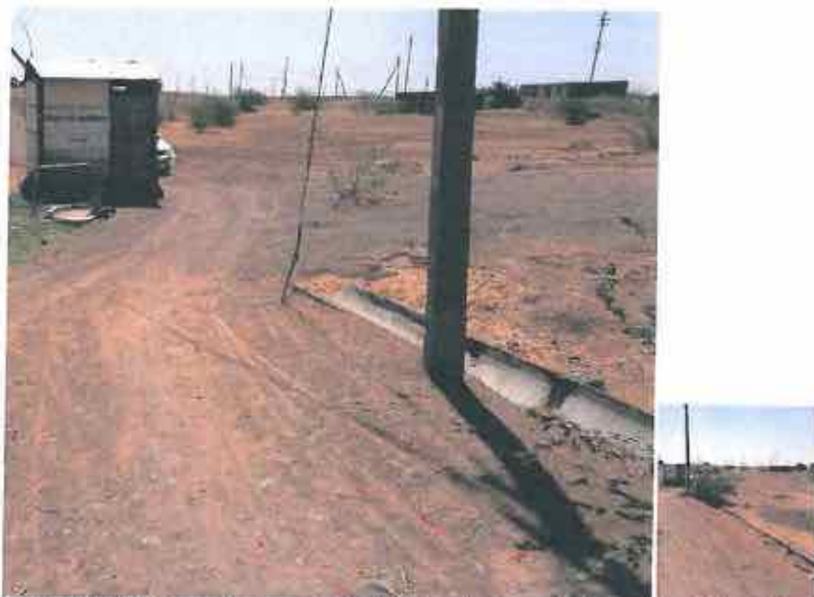
Ganpur Sirsi: Photographs of a semi-circular pipe drain coming from slope drains directly towards the Pumphouse some 6-7 m in front, posing risk of flooding of Tubewell and pumphouse during the rains.
