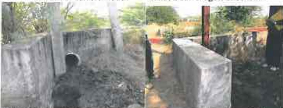
Chikalda: Two different poles PCC and HB constructed in front of Culvert
