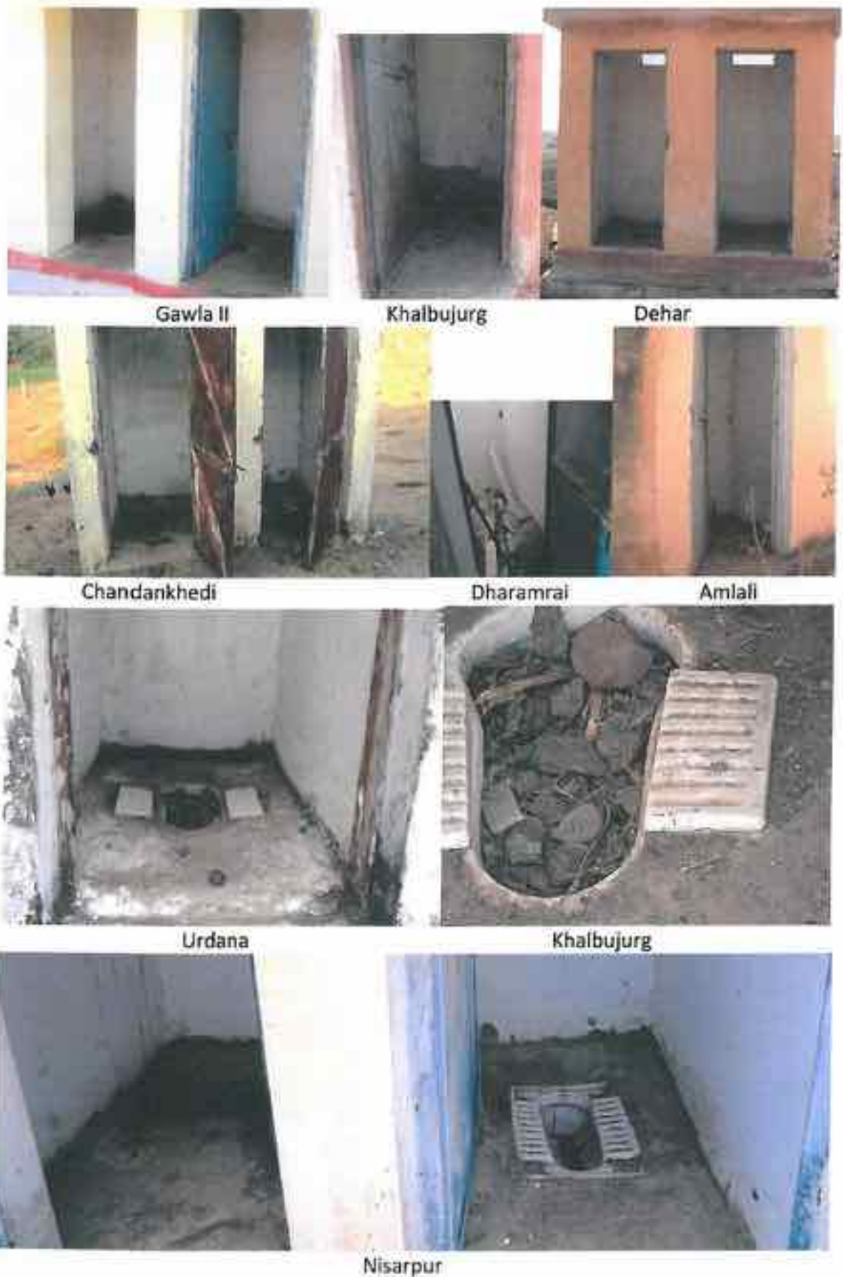
Plate 3.2.1. Dirty/stinking/unmaintained/unhygienic/defunct/out-of-use toilets without any provision of water and light. Typical for most buildings including Schools.
