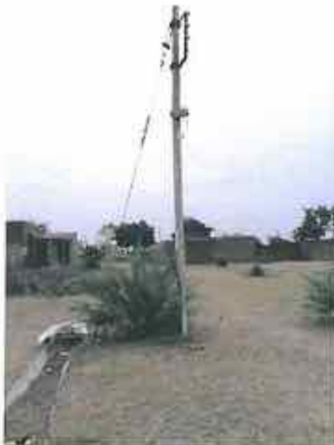
Sirsi Ganpur: Pole on road between road-side drain and road
