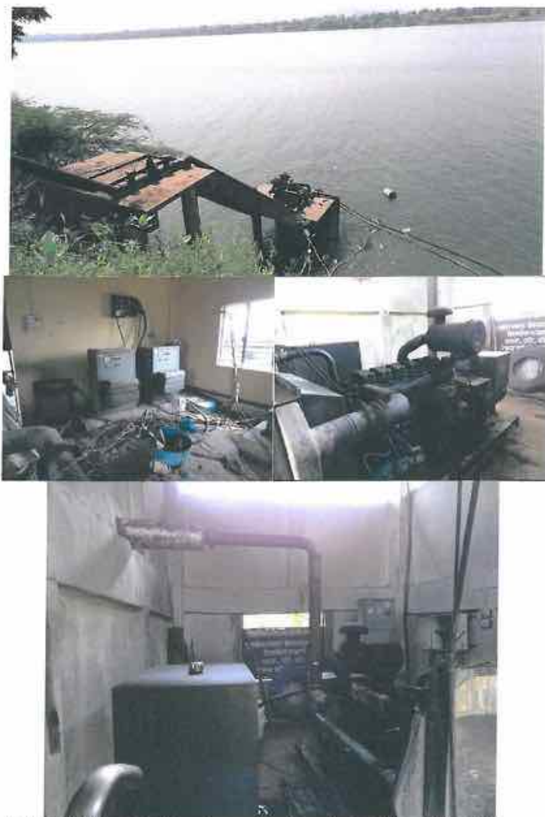
Plate 3.1.44. The Intake Structure and Equipment at Koteshwar Ghat, Nisarpur
