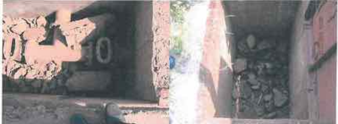
Brahmangaon Theekri (left) and Nisarpur(Right): Defunct, unmaintained, rubble inside
