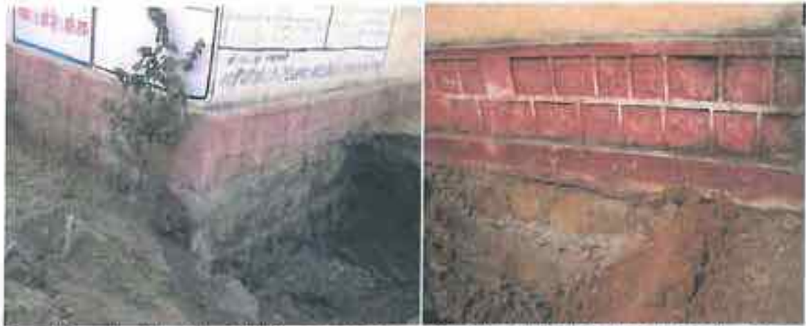
Foundation depth at Borlai II Panchayat Bhavan (left) with foundation depth 34 - 86 cm whereas at Kikarwas Primary School (right) foundation depth in similar strata was found 49-52 cm only.
