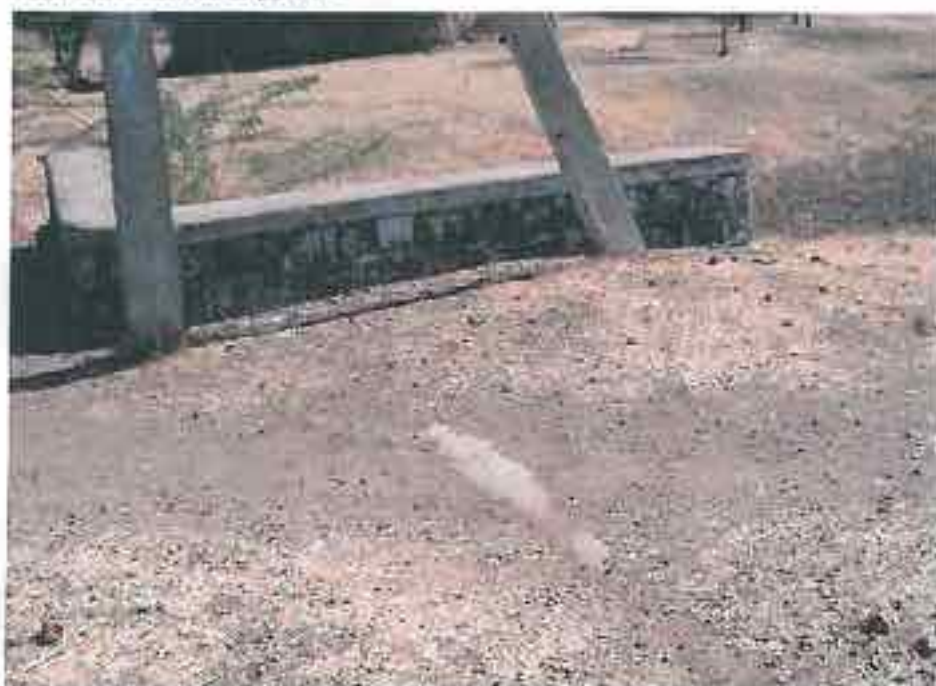
Borlai I: Cross drain pipes visible over roads: Inadequate covers on pipes
