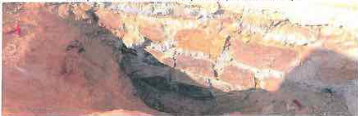
Chikalda-Panchayat Bhawan: Poor and thick joints-poor workmanship
