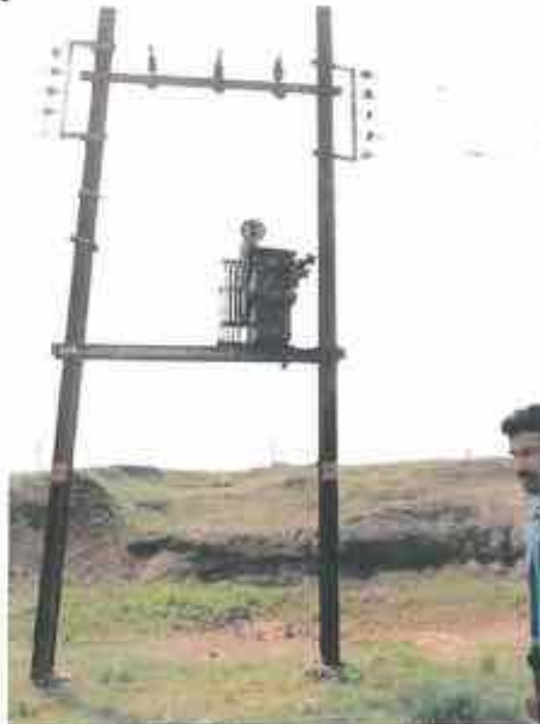
Nisarpur: LT Line taken from the 11 KV structure, which is not allowed as per safety norms. There should be separate LT pole so as to not energise the LT Circuit from the 11 KV Voltage due to leakage of current.
