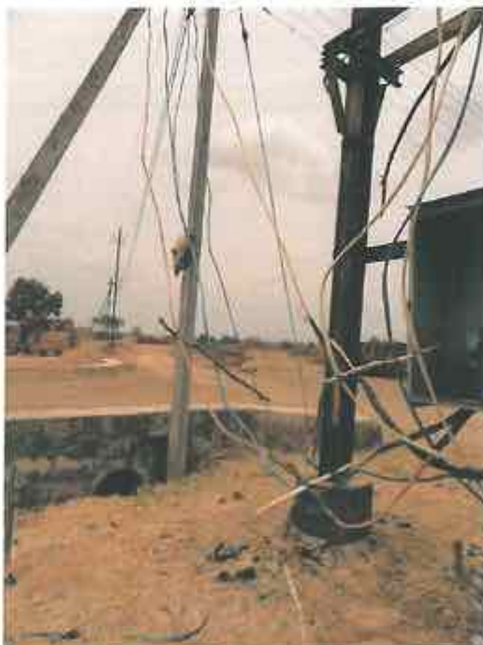
Tavlai Khurd : Poor pole location in front of culvert, Dangerous random spread of cables. Cable should be armoured and here armouring is missing. Cable found open which is dangerous to humans and animals. Poor maintenance also.
