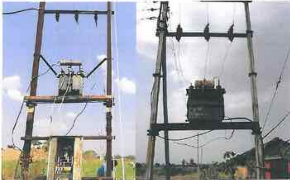
Typical Absence of AB Switches (Left-Moosapura(Dhar) and Right Kesur (Ramnagar))
