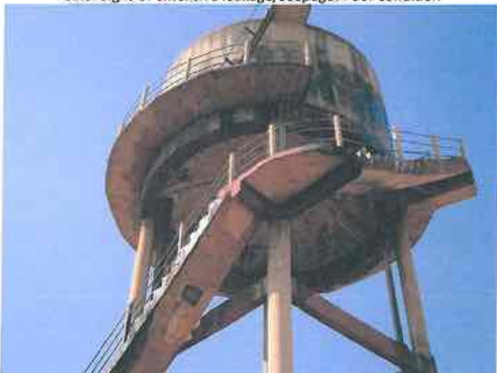
Sirsani: Extensive Seepage despite earlier efforts (whitish marks) at plugging the leakages
