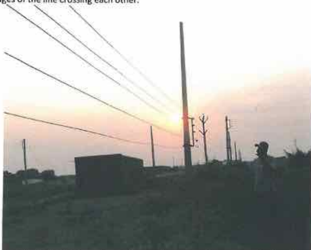
Nisarapur: Typical violation of minimum clearances above ground for the lowest conductors. Rule 77 of the Indian Electricity Rules, 1956, specifies a minimum clearance of 5.5 m for lines of medium and low voltages along any street (as is the case illustrated in photograph), 5.8 m across a street, and 4.6 m minimum for lines anywhere else.
