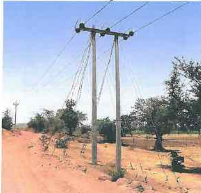
Plate 4.29. Vishwanath Kheda: When foundations are poor this is what may happen: As many as 10 guy wires seen supporting poles above which hardly has any load attached.
