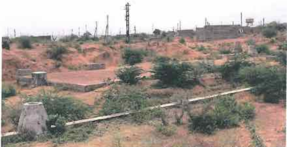
Plate 3.2.10. Dharampuri: One of the five massive septic tanks. In the front lies an encased sewerage line, and a big manhole, designed for low-lying area under flooding. If this sewer line gets flooded, it is very likely that the septic tank may also get flooded as well.
