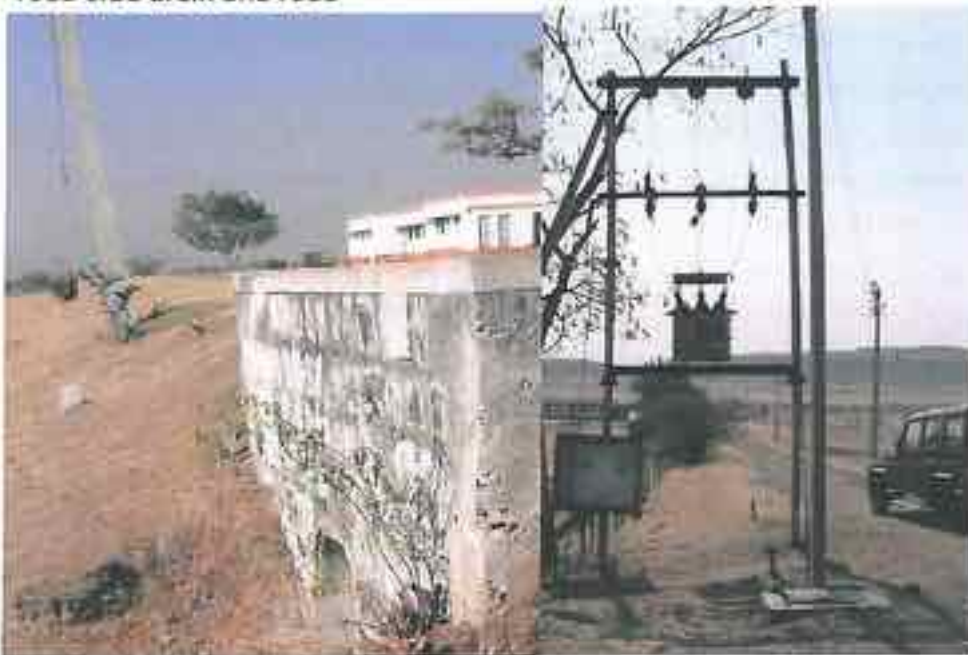
Dharamrai (Kukshi) Two different Poles encroaching upon Road shoulder/Road
