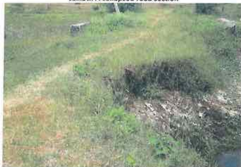
Moosapura: A damaged and collapsed road section.
