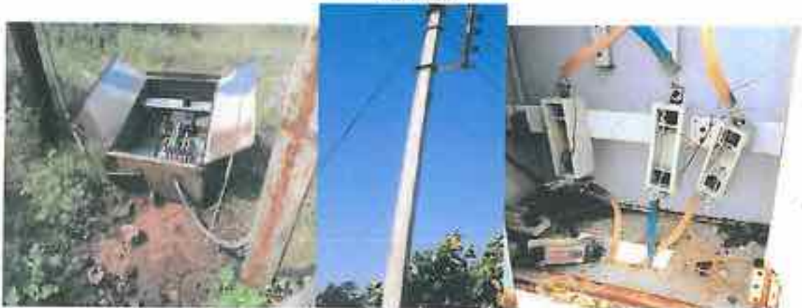
Niasarpur : LT-box on Ground Kavanthi: Broken Earthing Barda: Dangerous wiring
