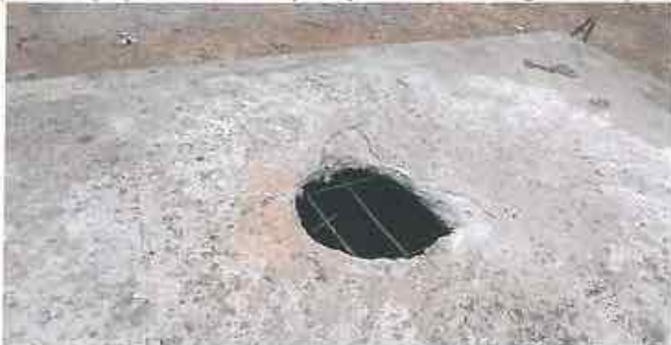
Beganda: Callousness in Construction: Septic tank Inspection/Entry chamber made as an afterthought after cutting the slab.
