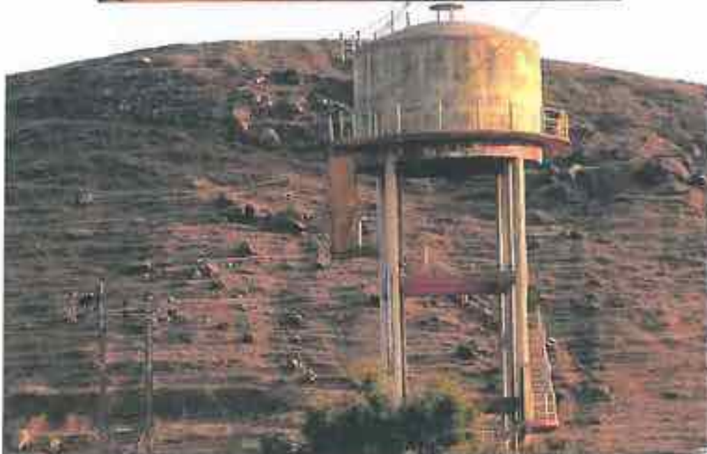
Sirsani: Missing fences, premises not marked and prohibited for public. Building lies too near. The OHT is located just below a hill where boulders lie loose, and may roll down damaging the OHT and risking the lives of people.
