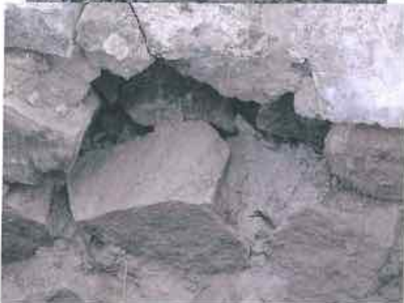
Chikalda: Primary School Building (left) showing typical foundation failure. Plate 2.1.21. Typical Foundation Failure
