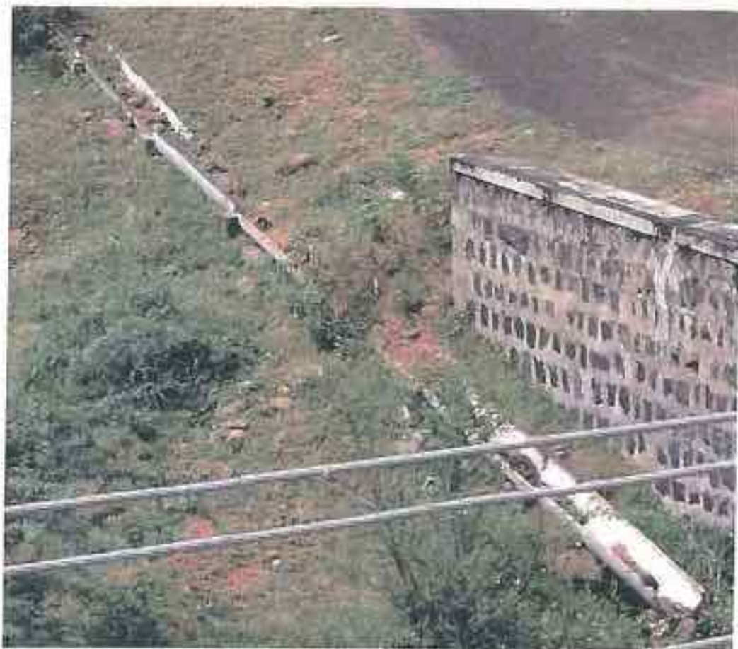
Nisarpur: Too steep profiles for pipe drains to work. The pipes joints are gone, and pipes are misaligned.
