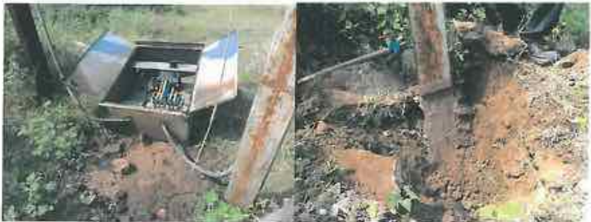
Nisarpur: Missing Muffings for two different poles
