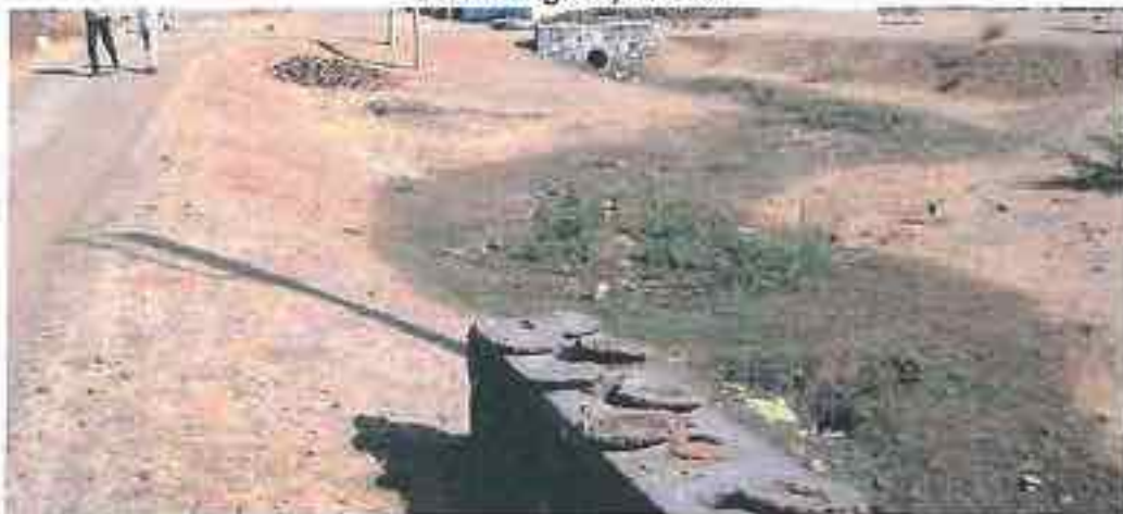
Borlai II water flows in zig zag pattern to find out the culvert made
