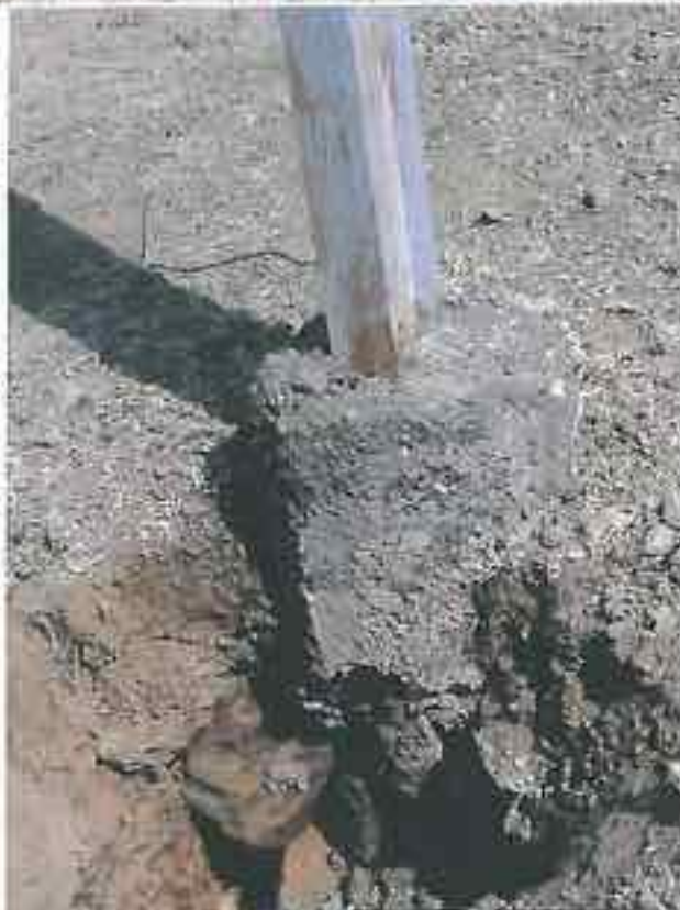
Plate 4.30. Borlai II Phase II - Metallic poles with recorded Concrete Foundations in MBs actually do not have even proper boulder foundations: Typical rampant malpractices – In some cases, muffings have been done away with (top photograph), while Cosmetic muffings provided in other cases to give an impression that concrete foundations lie underneath.
