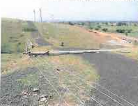
Nisarpur: Pole lying on Ground
