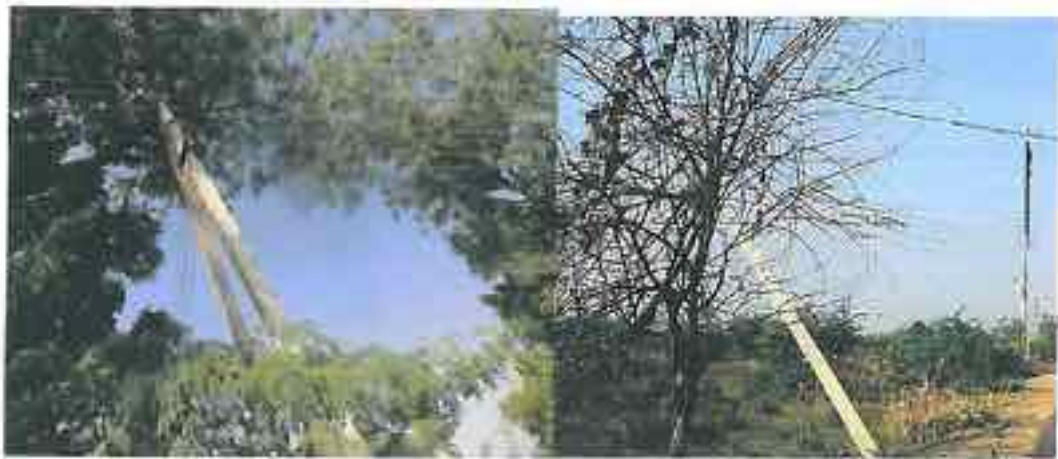
Tree clearances not maintained: Chikalda(Left) and Khalbujurg (Right)
