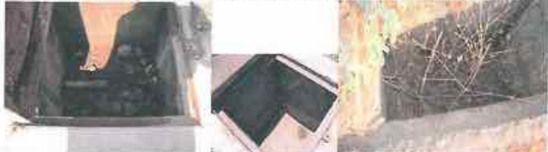
Amlali: Missing valves
