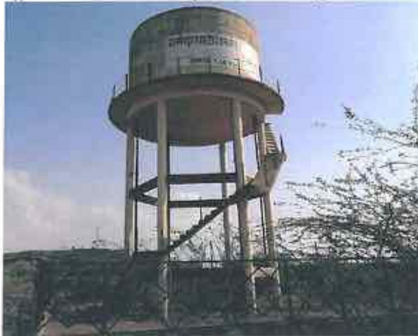
Gehalgaon : No provision of a sump for 150 KL OHT. Also note the missing railing.
