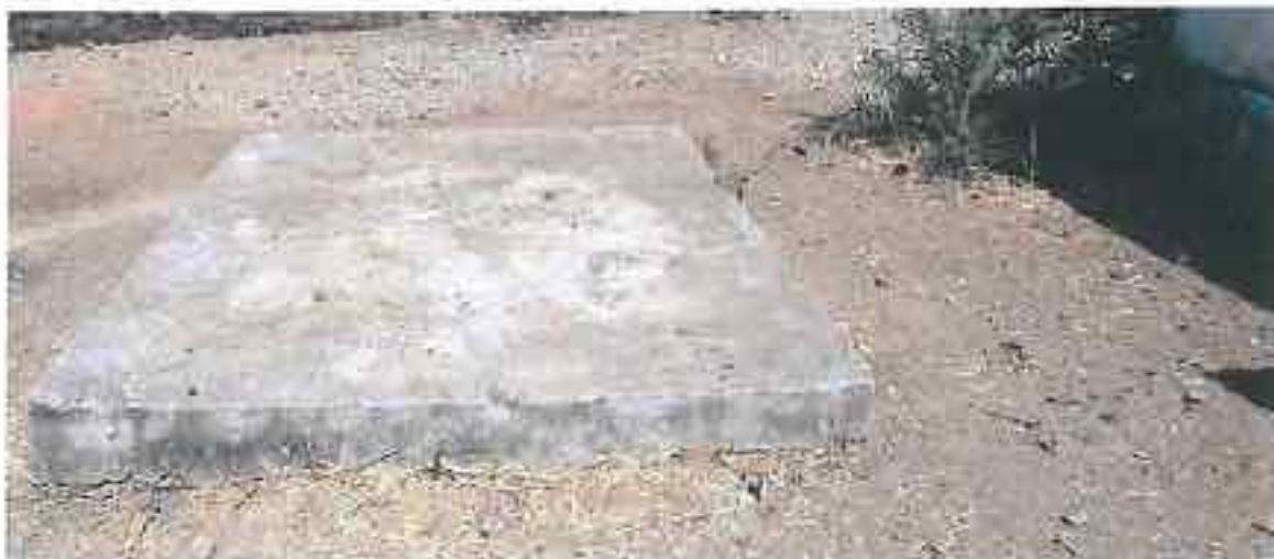
Chichli (Theekri) : Upper slab cast without any inspection opening. Inspection and Cleaning made impossible
