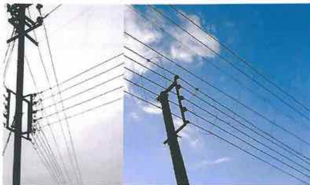
Broken Guarding wires touching LT conductors at Beganda (left) and Moreghadi (Right)
