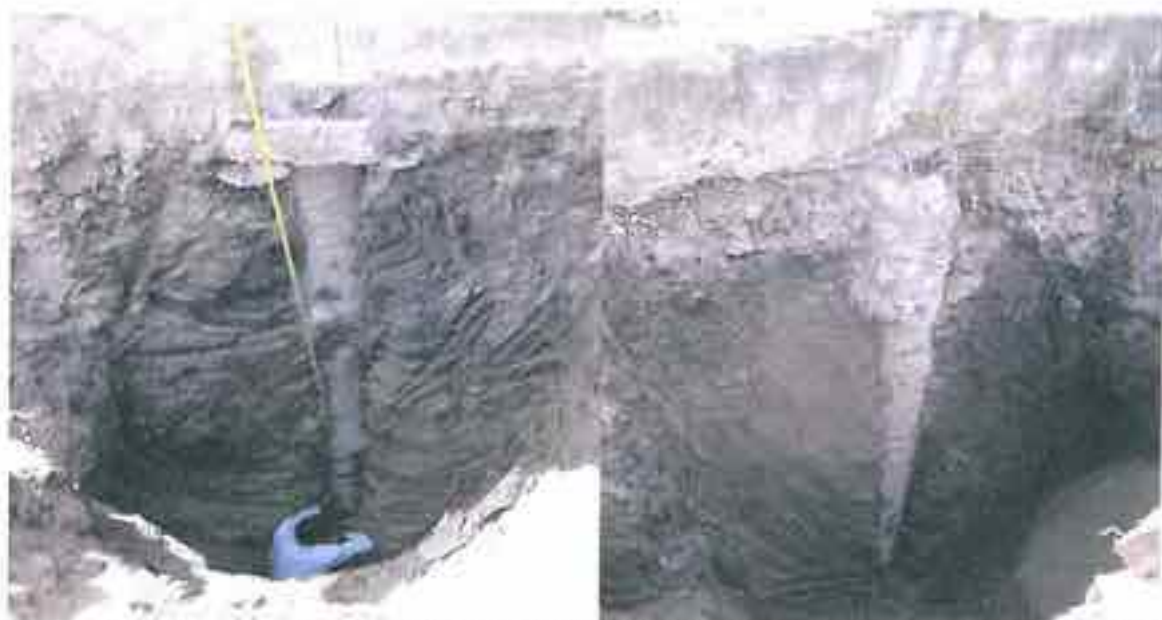
Noticeable pile eccentricity along the length (left), and shorter pile length (right) at Moreghadi Panchayat Bhawan. The depth of pile was found 20 cm short - as per MB it should have been 3.6 m, but pile measured only 3.4 m. Pile cap had a depth of 0.20 m.
