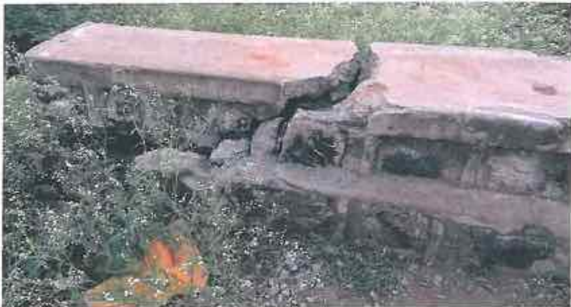
Ganpur: Foundation failure and poor workmanship of RR Masonry culvert
