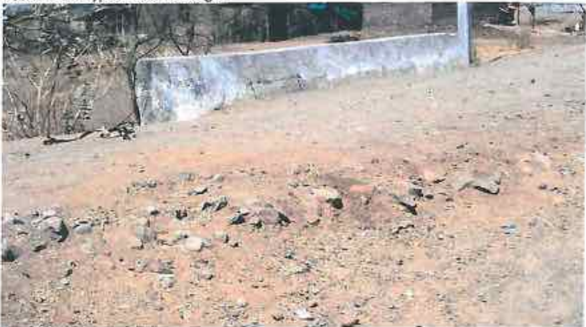
Gawla II: Typical road damages
