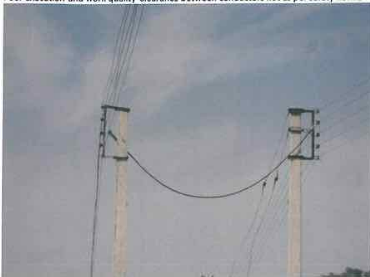
Missing Metallic Bearer wire to support cable: Poor work execution in violation of Rule 79 (2) of Indian Electricity Rules 1956
