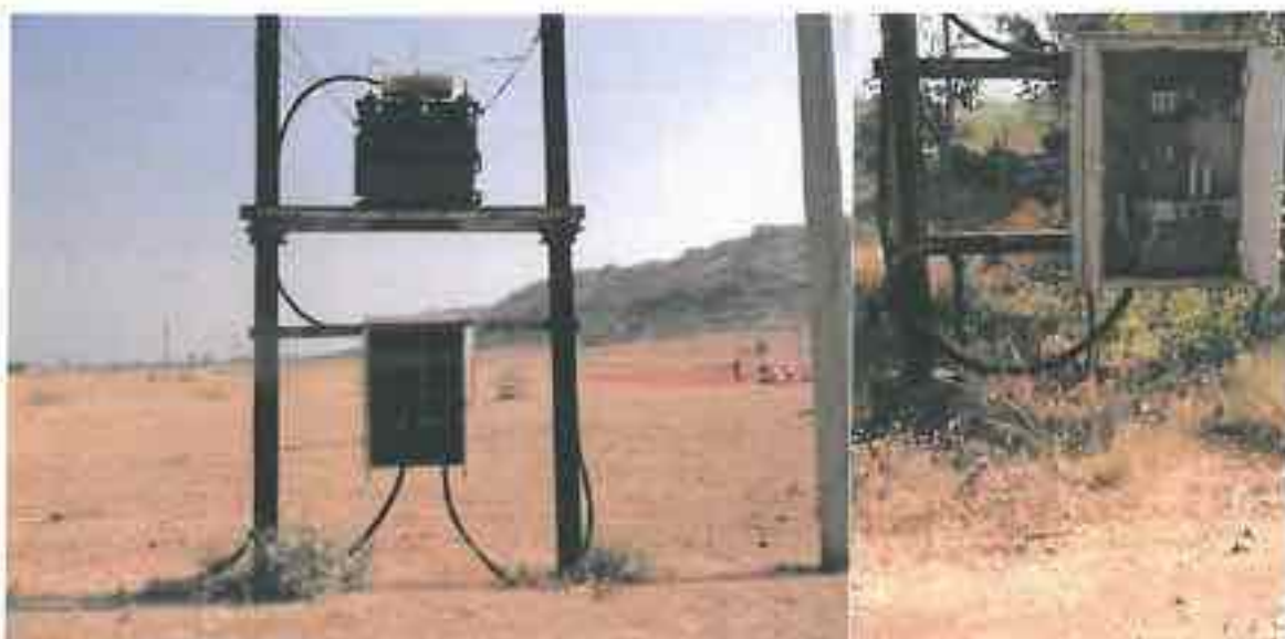
Plate 4.18. Borlai II, Phase 2: Inappropriate Ground clearances even in 2009 construction. Also seen are the missing muffings in the left photograph.
