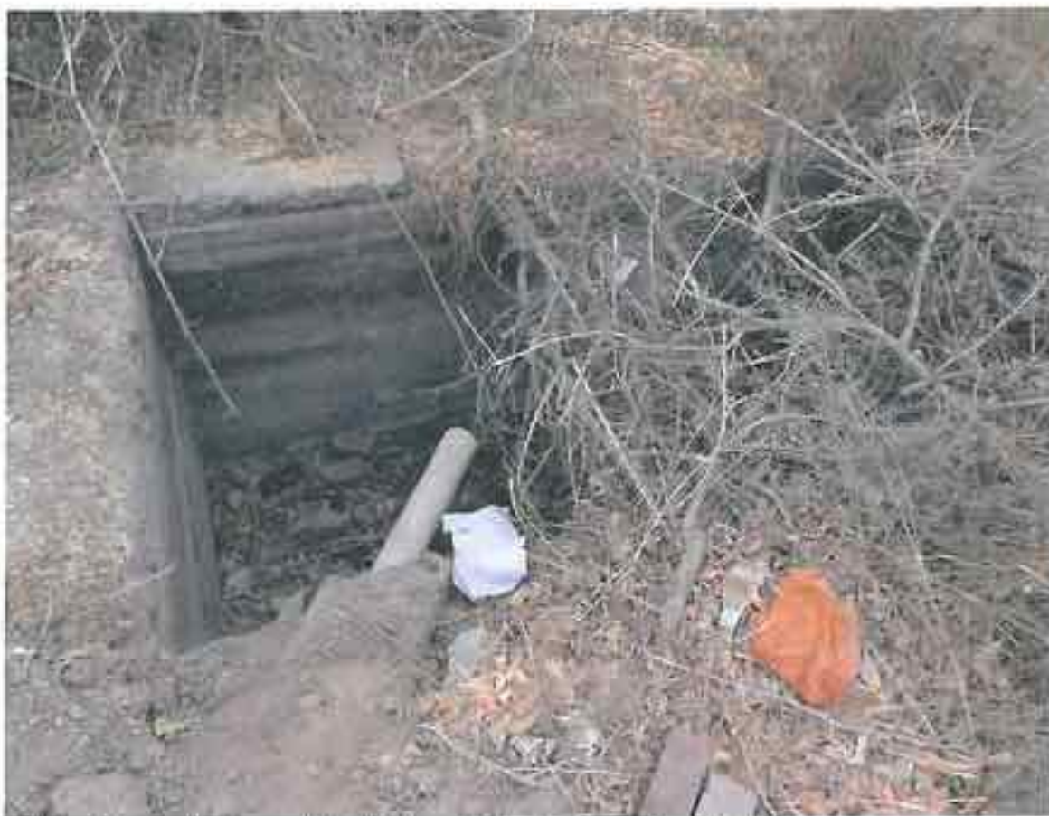
Golata: the whole upper slab of the septic tank not cast/not found
