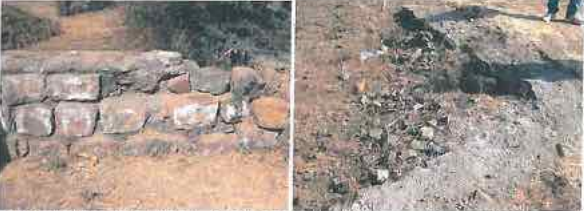
Jamda (left) & Borlai I (right): RR Masonry culvert with poor joints and inferior work quality
