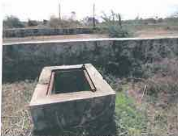
Ganpur (Narmada Nagar): Air valve Chamber, Cover also missing to facilitate immersion
