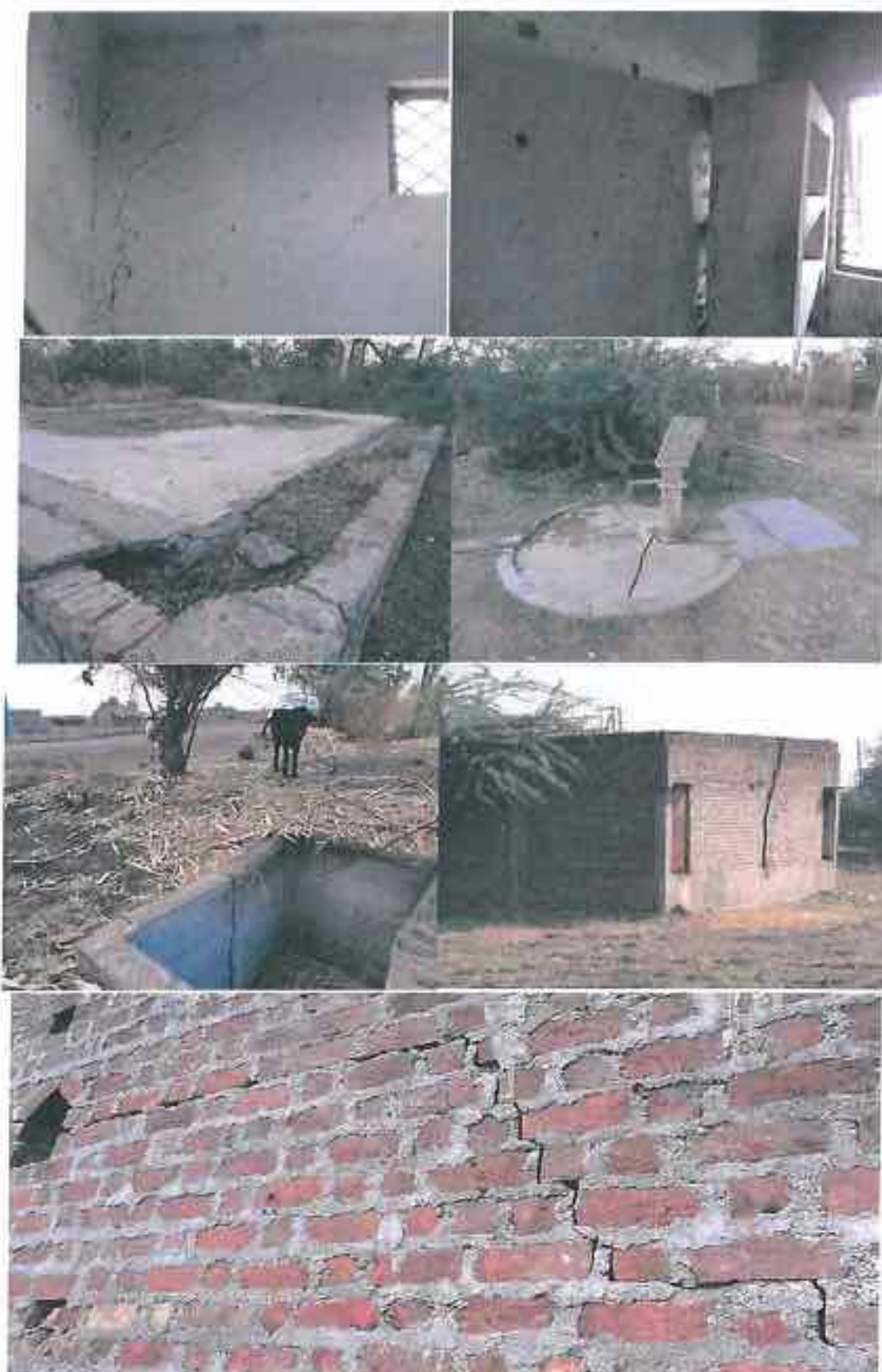
Plate 2.1.17. Construction in Prime BC Soil at Moreghadi and Khalbujurg: When the structures made by engineers have given way (top 4 photographs for Moreghadi), how will houses and structures of oustees (bottom 3 photographs) survive the onslaught of BC soil without any Technical help?
