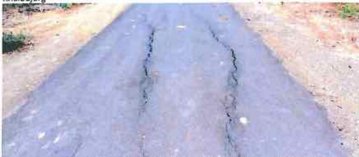
Dharampuri: Longitudinal cracks on Black Top BT Road- Typical of longitudinal crest failure and may be due to poor compaction in layers. Such cracks are also due to poor CBR of sub-surface and other layer material.
