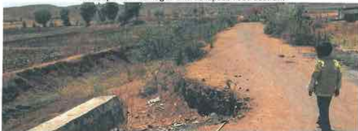
Chenpura: Typical Road damages
