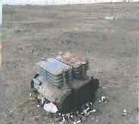
Khalkhurd (Dharampuri): Transformer lying abandoned on Ground
