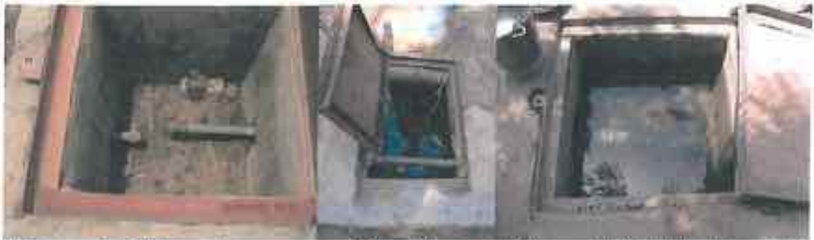
Dharampuri: Missing valve
