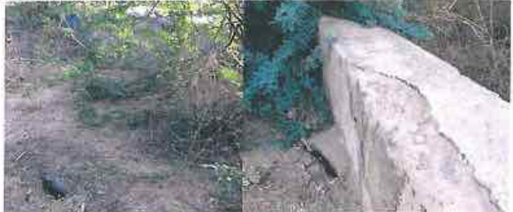
Saita (Kasravat) : 2 different Culverts with inadequate cover, if any.
