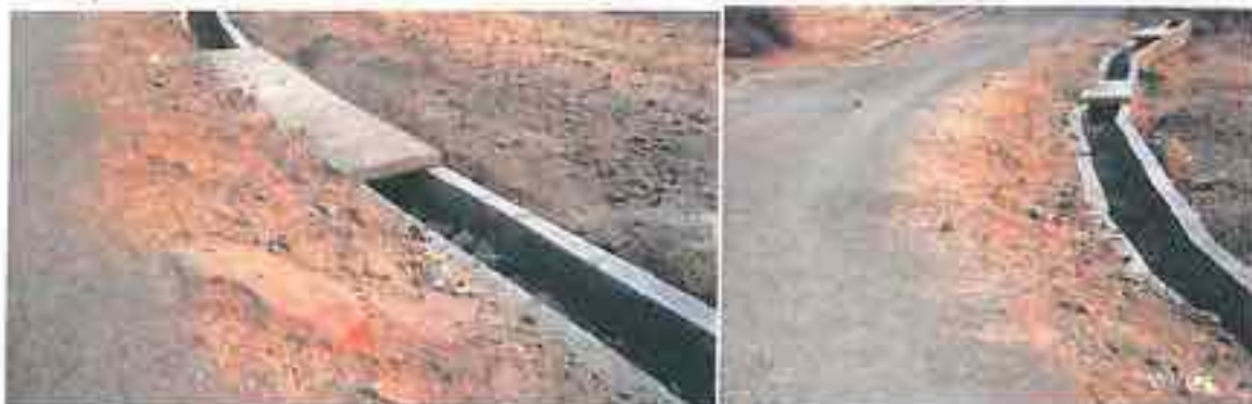
Mohipura: Boulder protruding (left)&Poor Road shoulders with wave-like drainage (Right)
