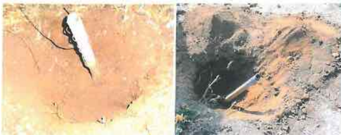
No Charcoal Seen in Earthings Typically at Jamda (Left) and Dharamrai(Right). Earthing connections not made according to IS:3043-1987.
