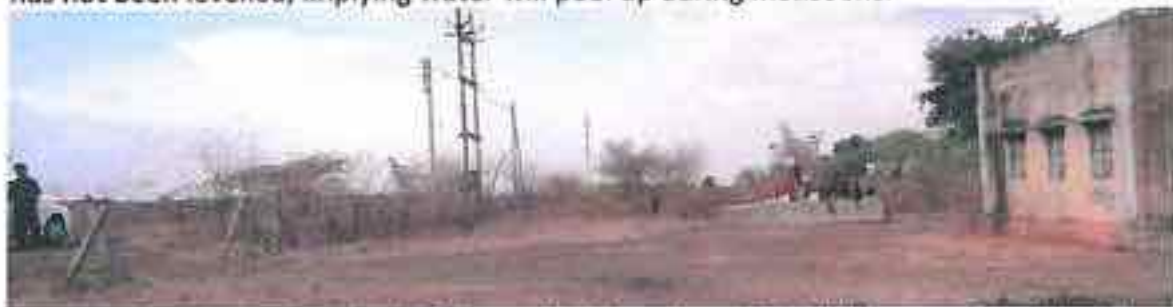
Moreghadhi: The road at the left is much higher than the building premises. Plinth has not been raised appropriately relative to road formation.
