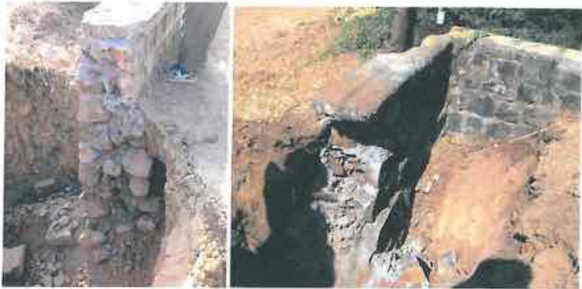
Amlali: RR Masonry Culvert. Poor workmanship and quality. Culvert pipe mouth seen blocked, and how water will pass through is beyond imagination. Upstream ground level is above road formation level, so water is overtopping road formation rather than pass through culvert pipe
