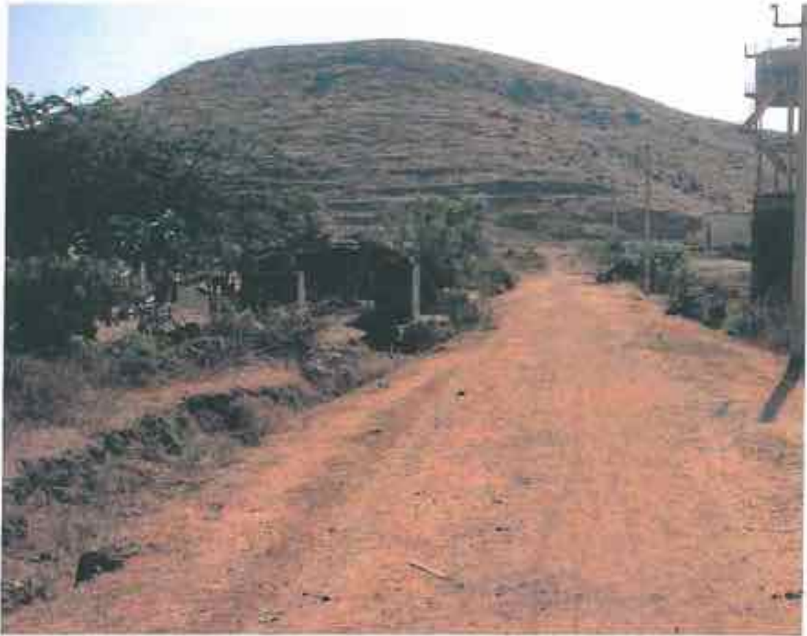
Sirsaani: Deep trenches alongside the road. Are these trenches made during construction by use of soil therein?
