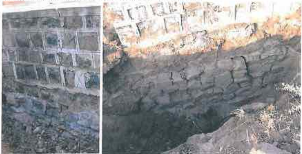
Foundation of Tree Platforms showing poor masonry joints leading to vertical cracks at Eklera(left) and poor and almost non-existent masonry joints at Khedi Bagood (right).
