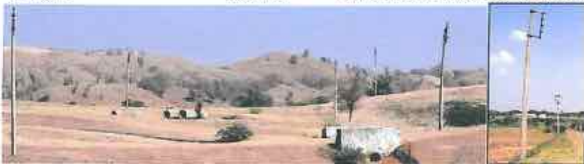
Poles not having straight profile: bent visible Kikarwas (Left) and Moosapura (Right) Plate 4.31. Poor PCC Pole qualities
