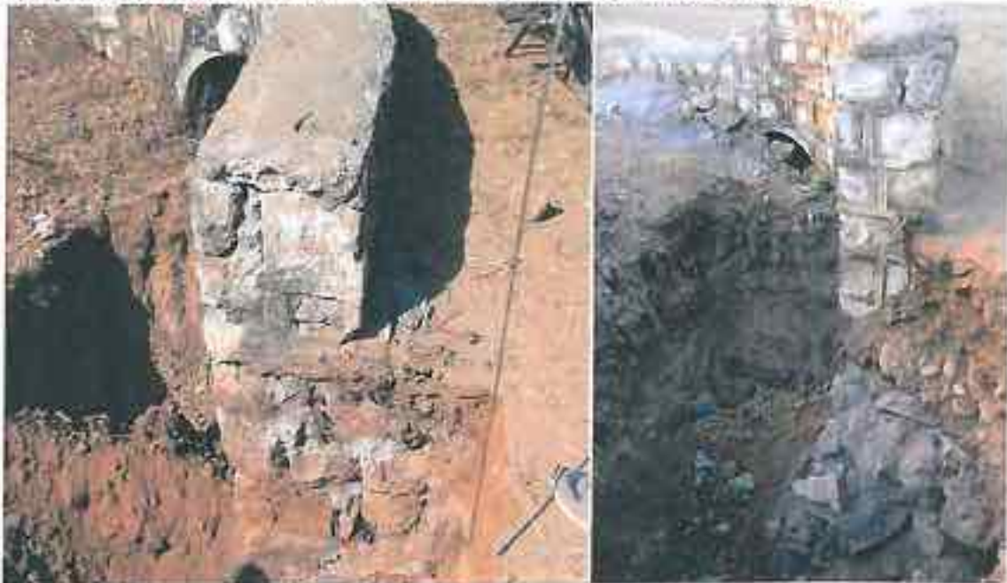
Jamda (left) and Kalyanpura (right) : RR Masonry culverts with poor quality of work
