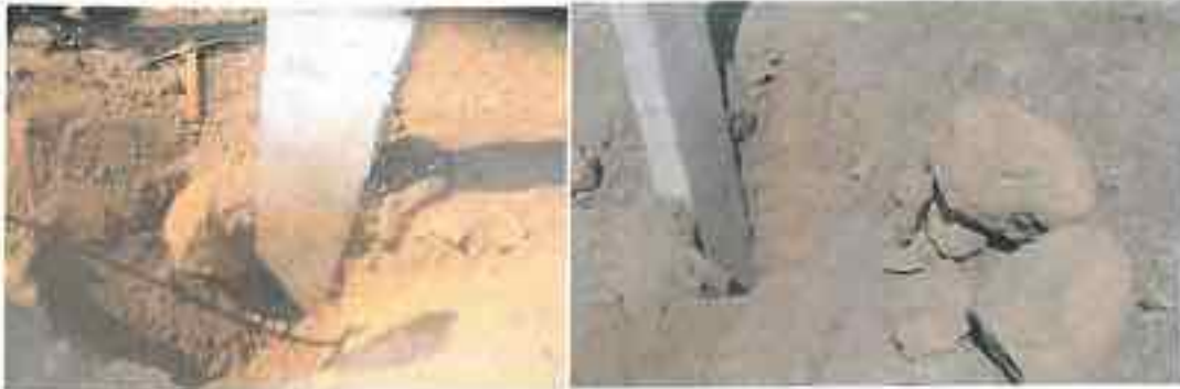
Dharamrai: Inappropriate poor Packing
