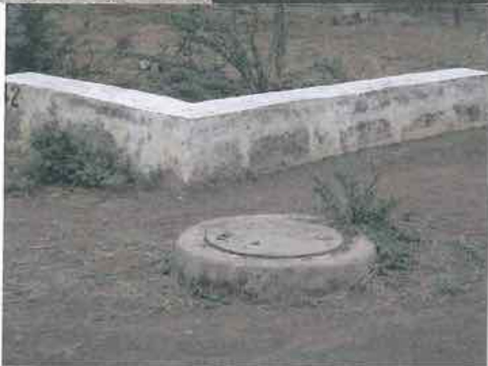
Plate 3.2.11. Dharampuri: Typical Manholes rising above road level. Safety jeopardised.
