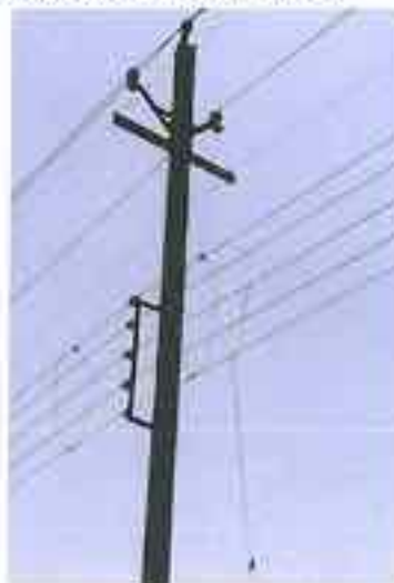
Plate 4.42. Lakhangaon: Makeshift arrangements to get streets lighted by hanging bulb
