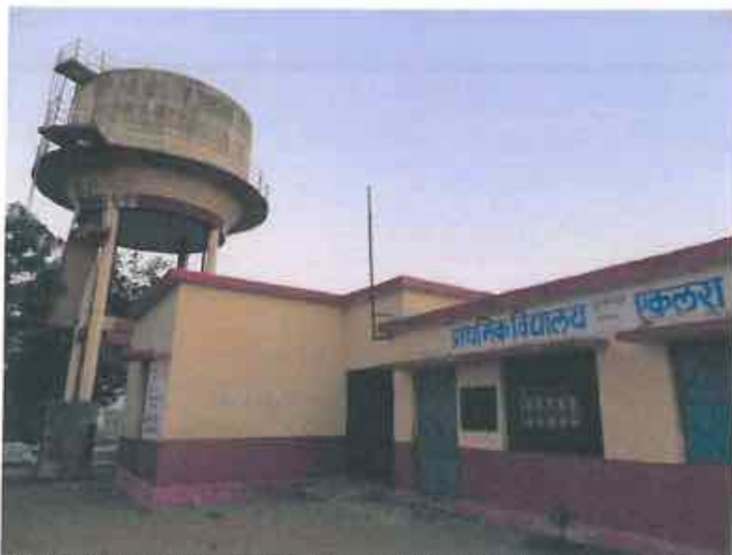
Eklera: OHT located in the premises of Primary School. No fencing present either for the school or the OHT, implying free access for the school children.
