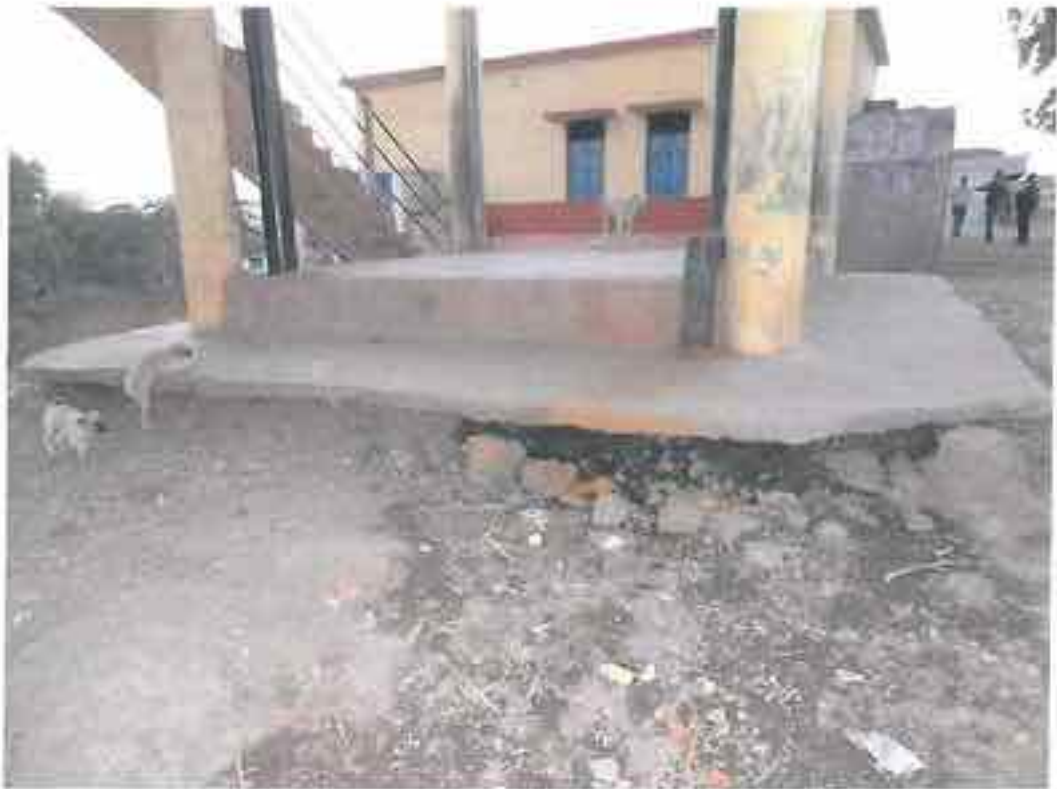
Eklera : Damaged Base Platform for an OHT located within 10 m of a Primary School (seen in the background)
