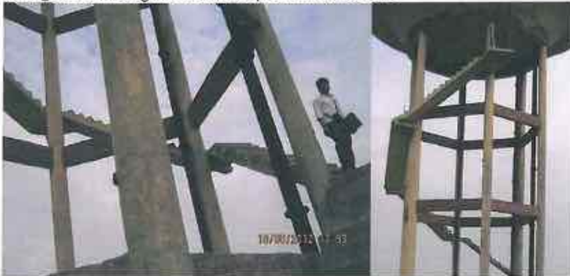
Khalkhurd (Manavar): Completely missing Railings, No gate: Easy access
