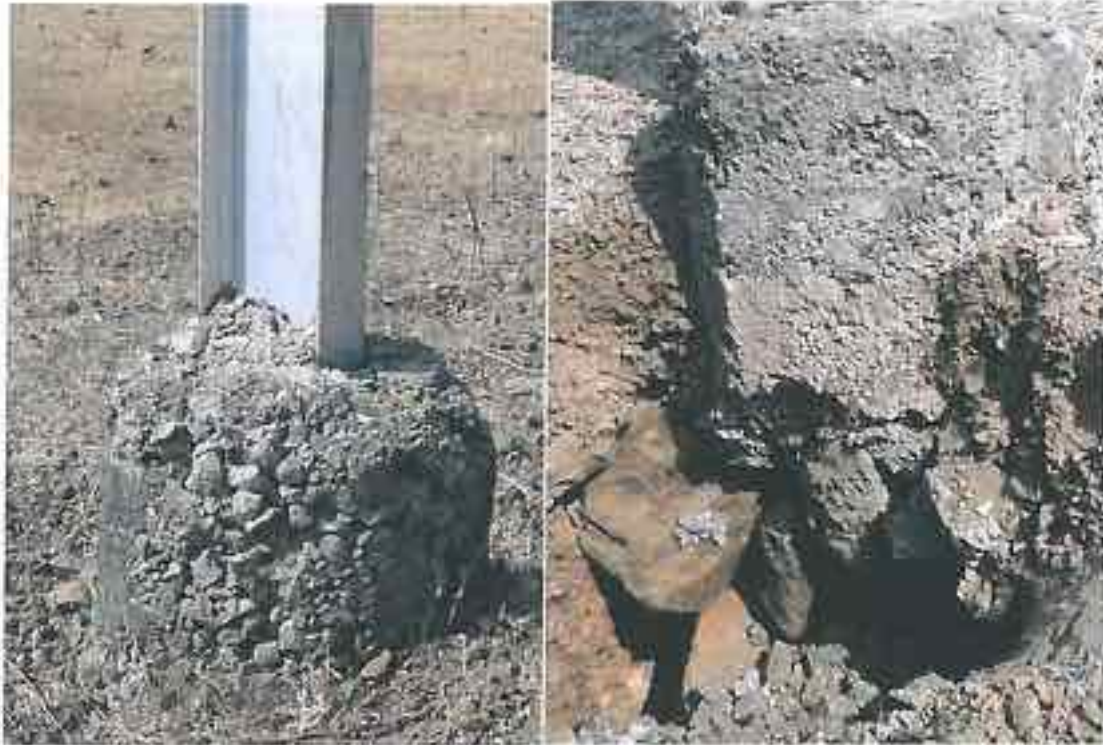
Very Poor quality of concrete in Muffings
