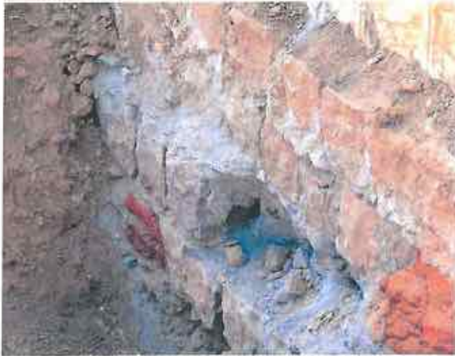
Amlali: Foundation of Panchayat Bhawan- Poor joints
