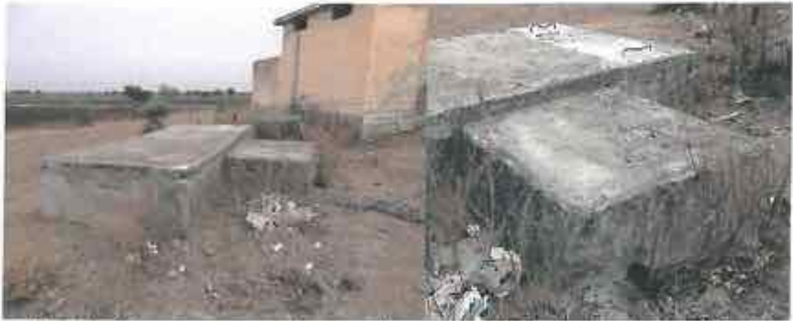
Beganda: No proper cover at the top—inspection and cleaning made very difficult
