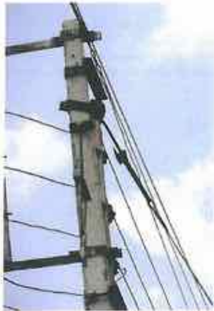
Mirzapur: Conductors directly tied
