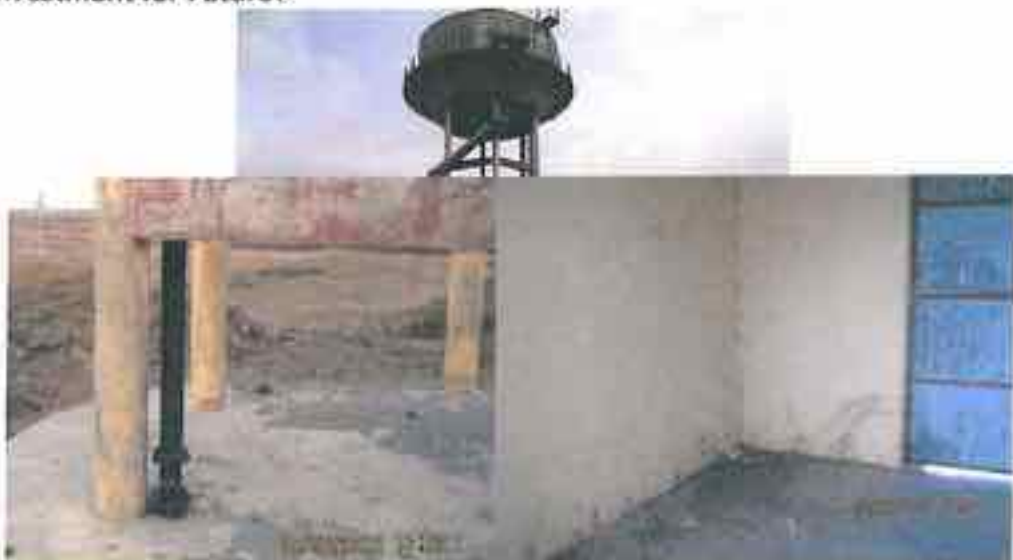
Khalkhurd Manavar: OHT built, but has missing Connections and Pumps
