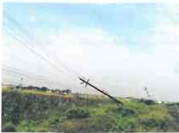
Nisarpur HB Poles
