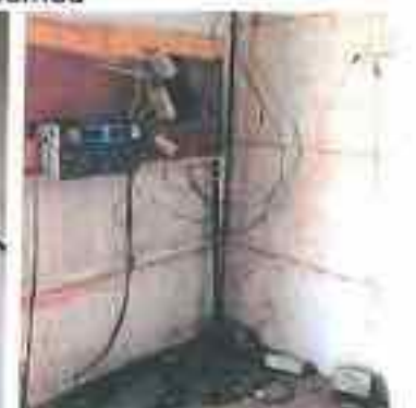
Ganpur Sirsi: Meter thrown on floor & direct connection made
