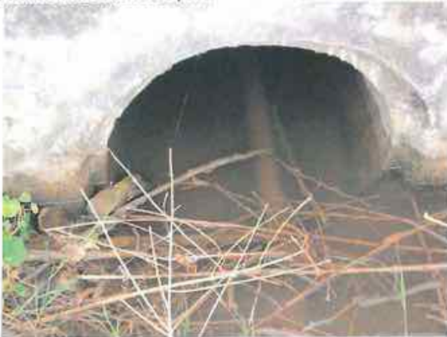
Ratwa: Water supply pipe submerged in flooded culvert dirty water
