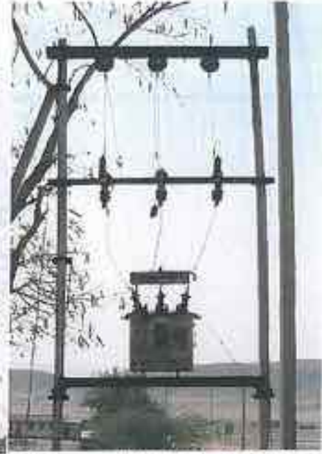
Dharamrai (Kukshi): only 2 LAs present, 1 seems burst, Also Placed Inappropriately
