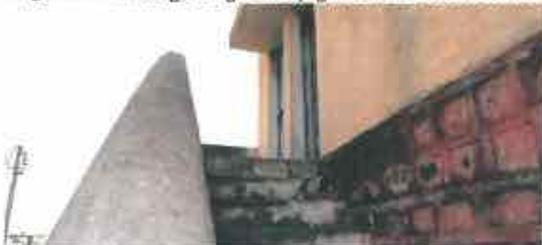
Nisarpur...The toilet pipe discharges to footsteps!!...
