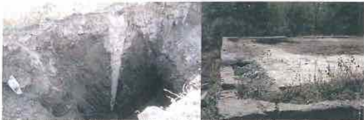
Moreghadi: Typical 2.77 m deep pile foundation (left) for tree platform in the premise of overhead tank. This platform was seen in very poor state (right). The pile depth of 2.77 m had no design basis. The quality of work was also very poor.
