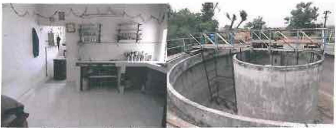
Dharampuri: Plant not working, lab was not found equipped, Treatment Units found empty and dry.
