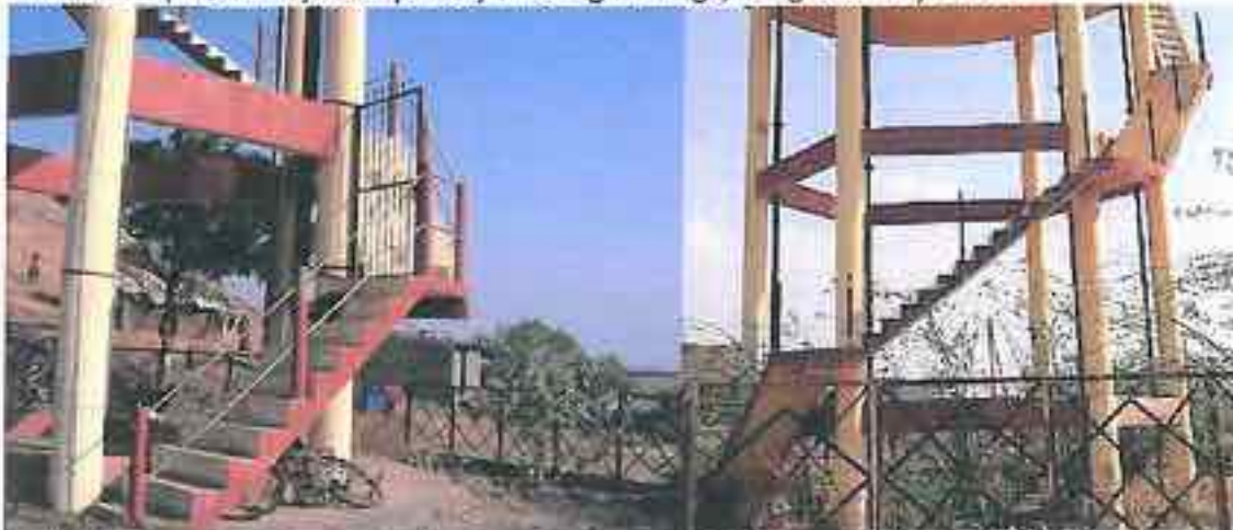
Borlai II: Premises fenced, and gate present on steps to prevent easy access to the top. And yet, the railing is only on one side of the steps.
