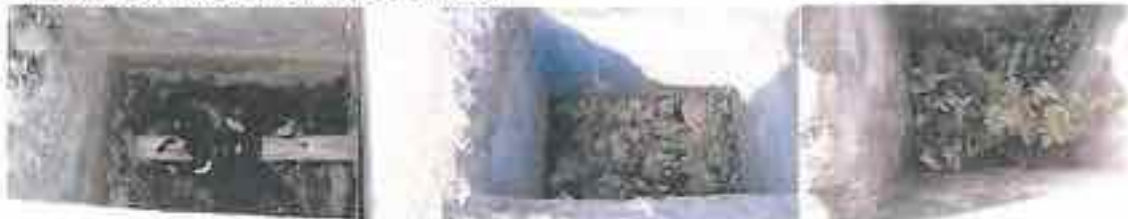
Awalda: Missing valves, broken connections, rubble inside Takiapur: Vegetation inside
