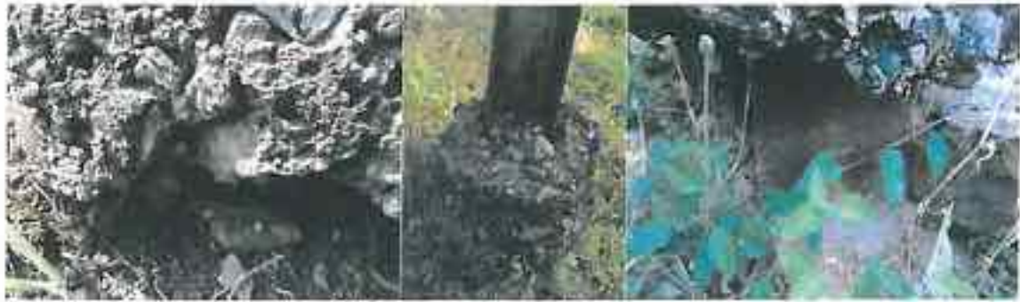
Very Poor concrete quality: 3 different poles at Nisarpur
