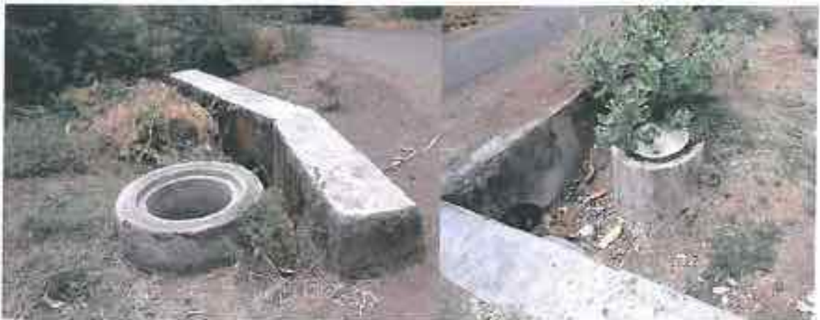
Plate 3.2.12. Dharampuri: Typical Manhole Locations with respect to Culverts. Note also the missing cover in one case.
