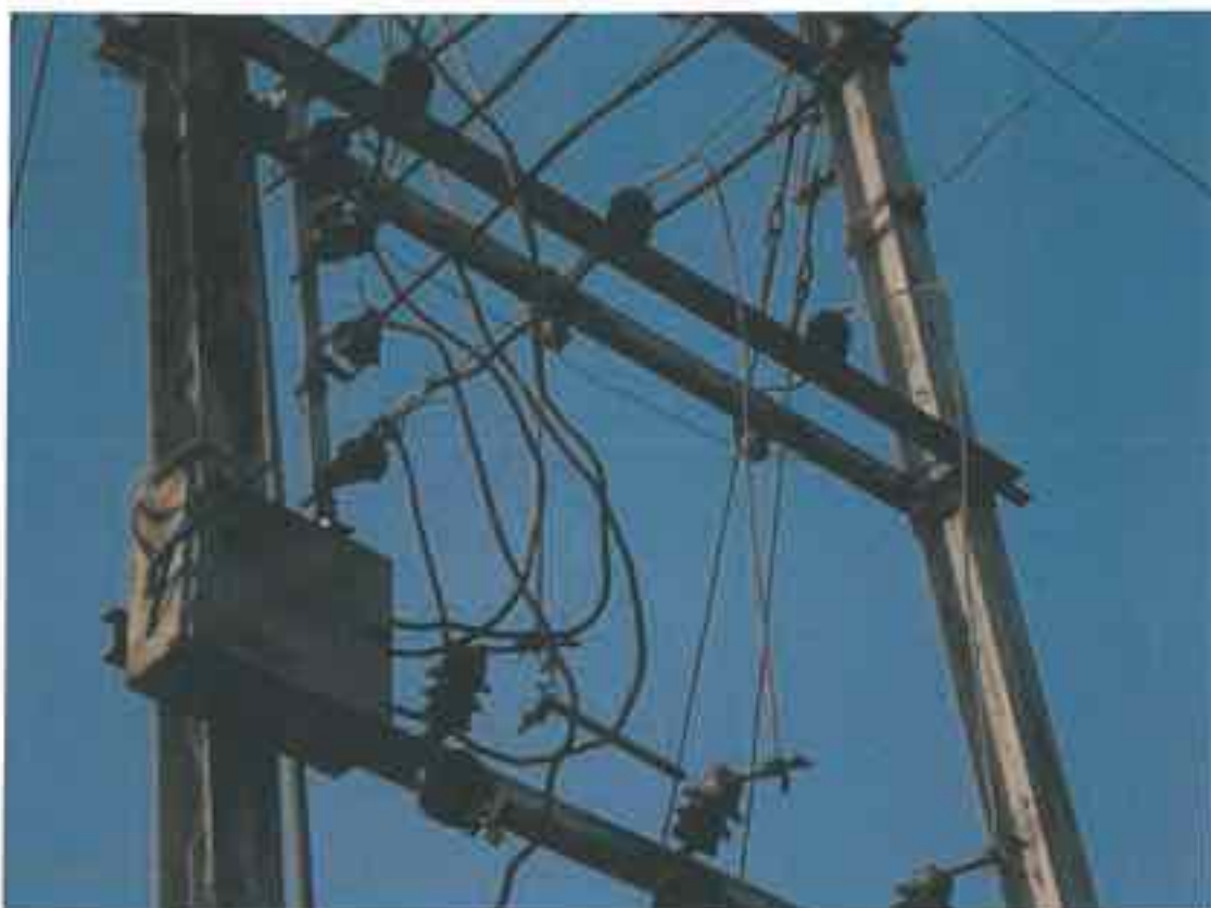
Poor execution and work quality-Clearance between conductors not as per safety norms
