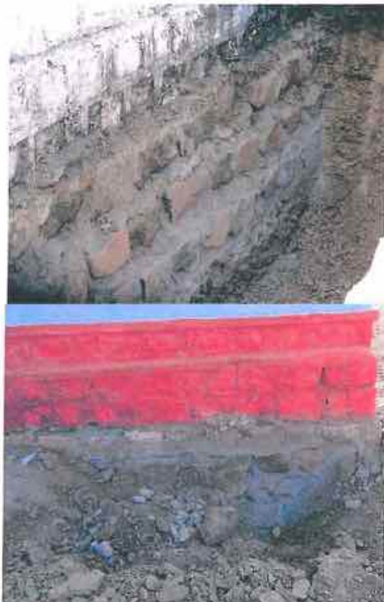
Bolai I Primary Health Centre (Top) & Morekatta School (Bottom) showing poor and thick masonry joints
