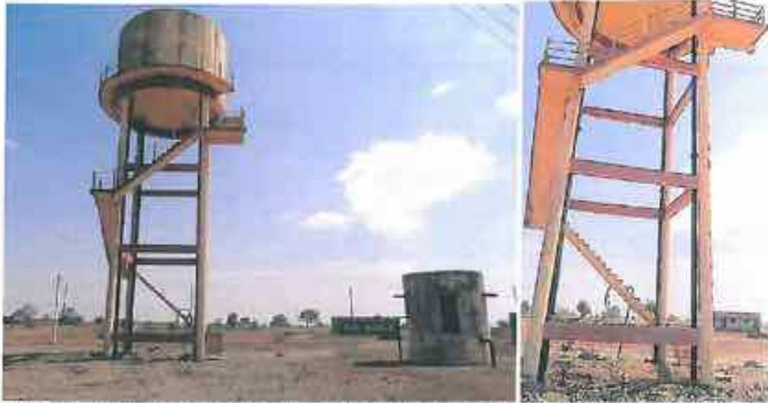
Ganpur (Manavar): No fencing and isolation of OHT Premises. OHT railing also partly damaged and missing in the lower steps: Poor maintenance
