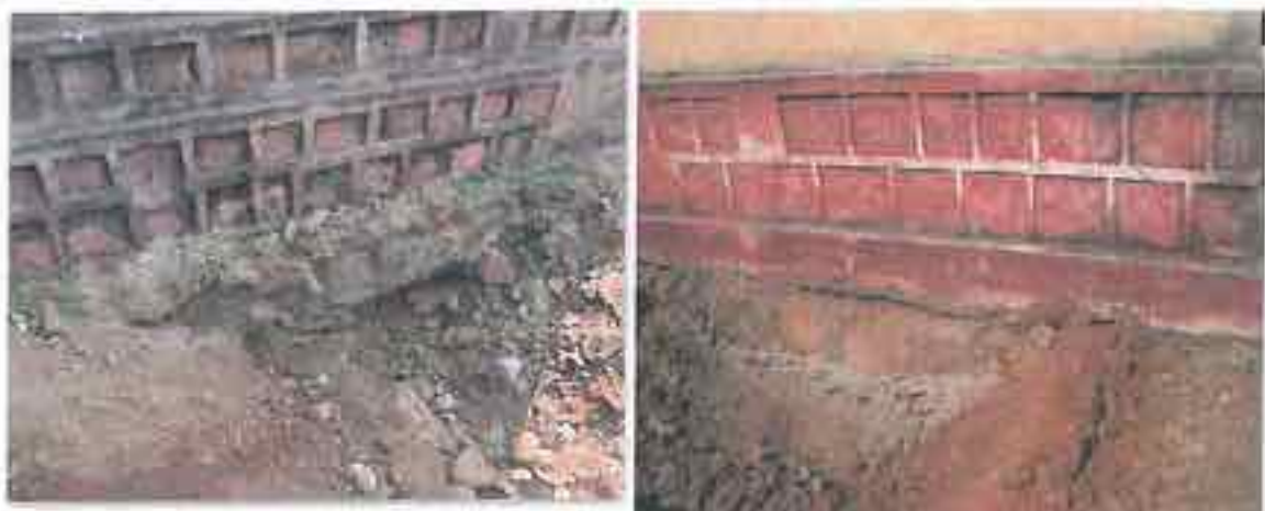
Foundation of Middle School Building had only 40-61 cms depth at Nisarpur I (left), whereas in similar strata at Primary School Kikarwas (right) 49-52 cm deep foundation was provided.
