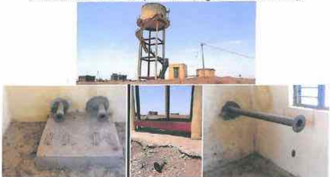
Kadmal: OHT stands tall, but missing Pumps, Connections imply defunct Infrastructure
