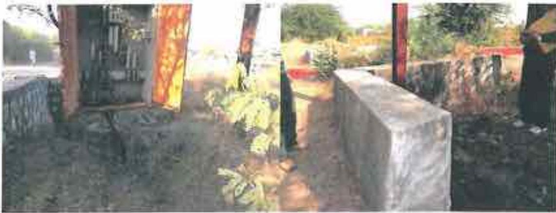
Bhilkheda: Transformer Switchboard panel
