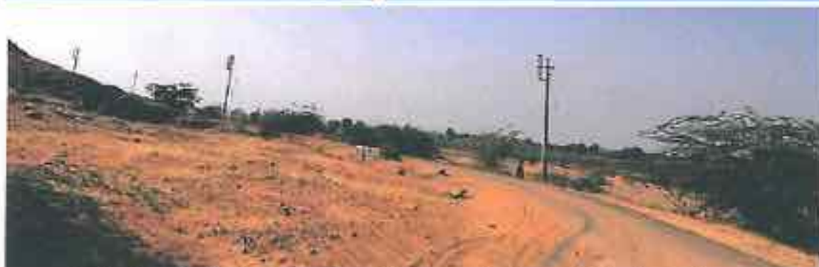
Balwada: Shackle insulators provided at turning instead of split insulators
