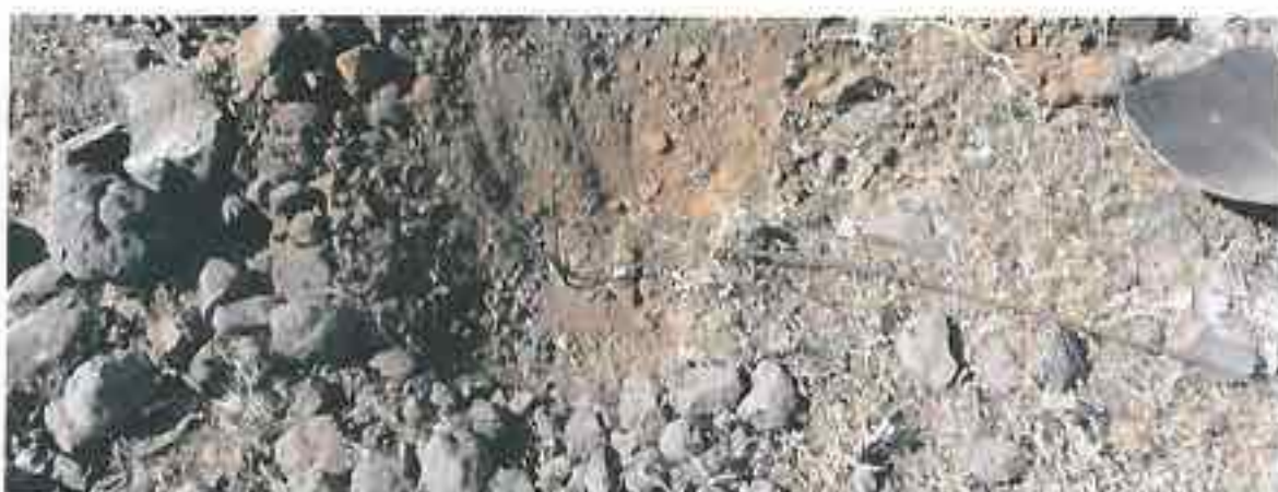
Dehar: Earthing wires without GI rod
