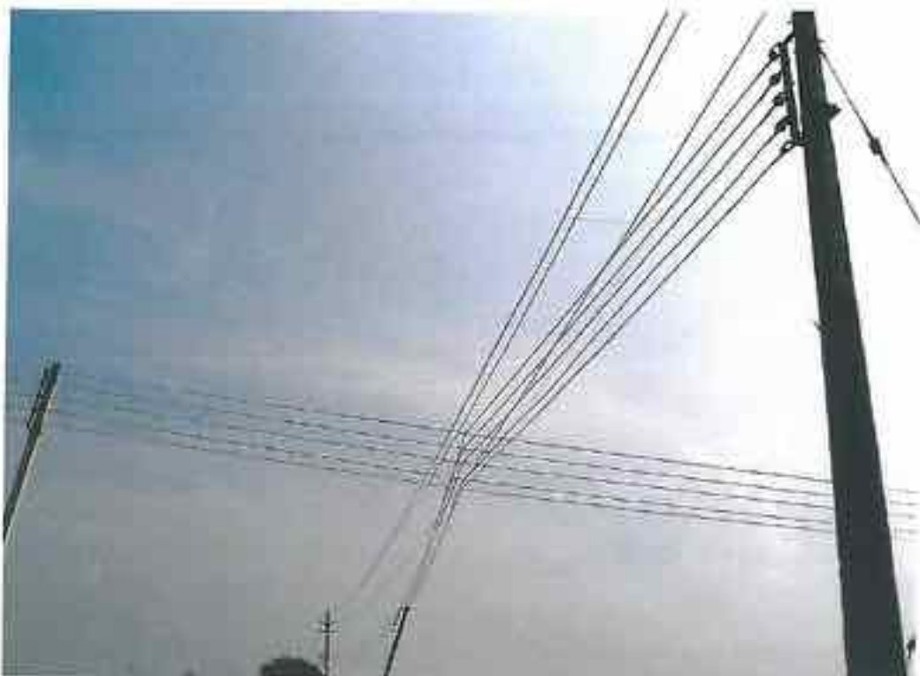
Nisarapur: Violation of Rule 87 (3) of the Indian Electricity Rules, 1956, which requires 2.44 m (at the very minimum) or more of the minimum clearance depending upon the system voltages of the line crossing each other.
