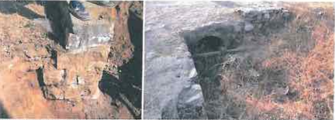
Poor quality of workmanship with poor masonry work at culvert foundation at Bhawti II (left) and head wall of RR Masonry culvert at Dharamrai (right)
