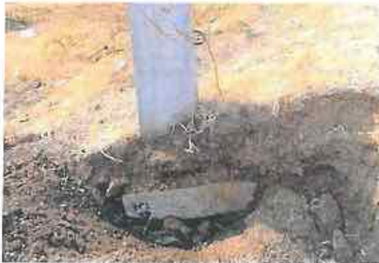
Plate 4.27. Borlaj I: Improper random packing, even readily available marking stones for plots (here plot no. 43 as evident) used as pole base packing
